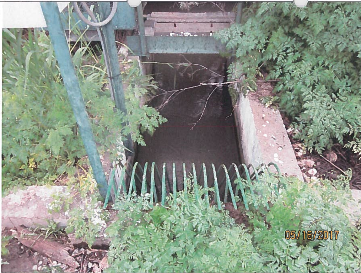
Concrete box that directs water to the pond.
