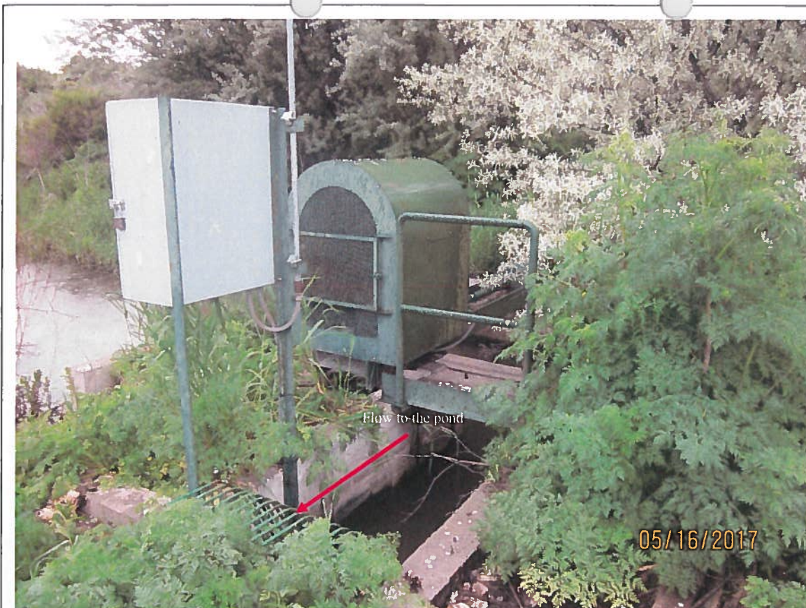
Control Gate that adjusts flow in the Canyon County Ditch #2. Raising the gate dams the water and allows flow to the pond.
