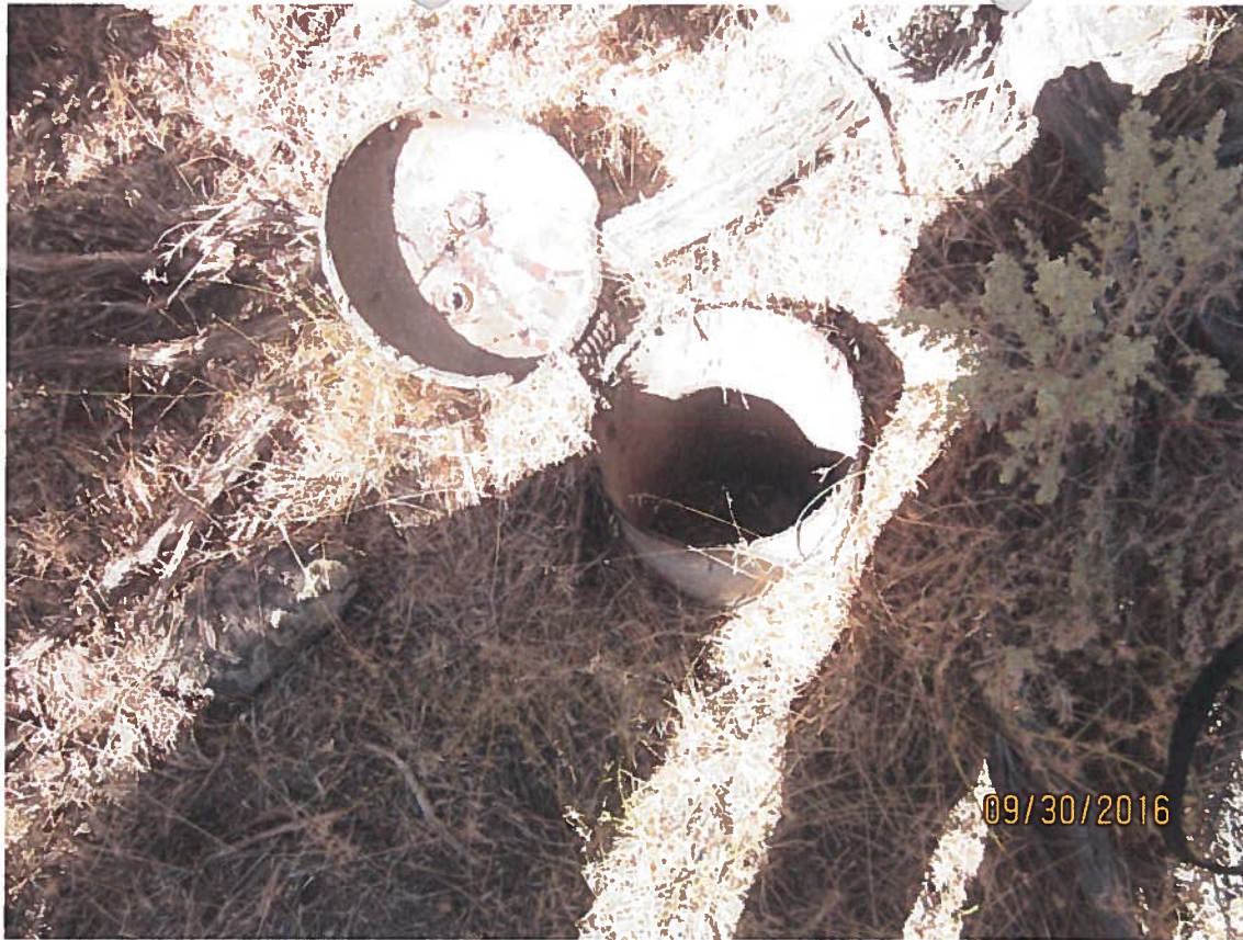
Valve box used to turn the water on/off at the main line.
