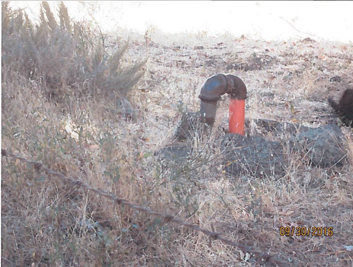
Air vent for the three springs that connect to the main irrigation line. This is found in the SESW QQ of section 2.
