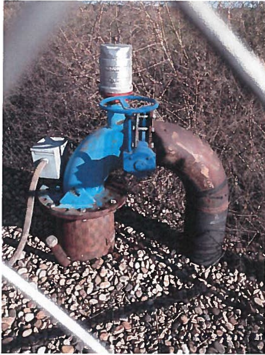
Figure 1 The 16" well diverting water to the concrete box to the north.
