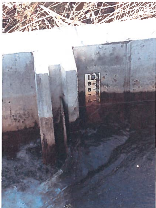
Figure 3 The staff gauge and cipoletti weir in the concrete box north of the well. The picture was taken before the water level reached an equilibrium. Water can be diverted either west or north from the box to flood either of the two cells.
