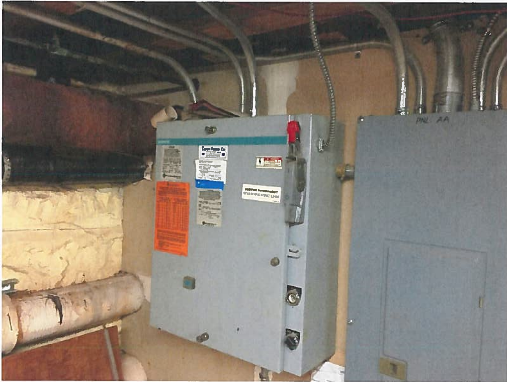
Well 1 Pump Control Panel
