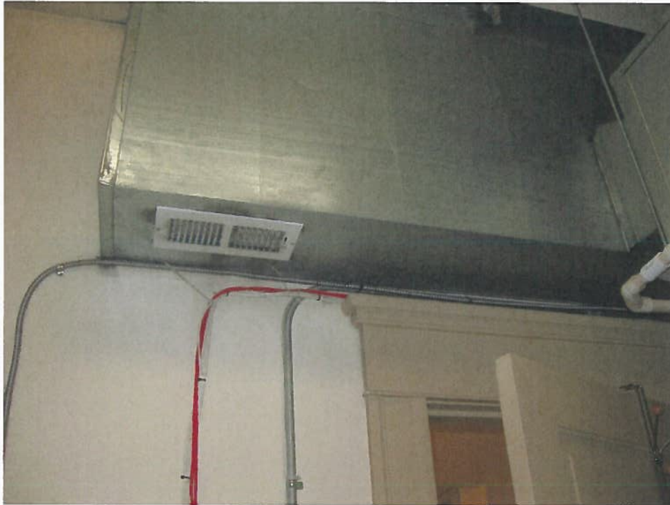
Sample Cooling Unit
