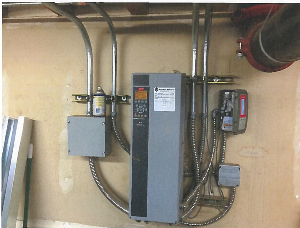
Well 2 Pump Control Panel
