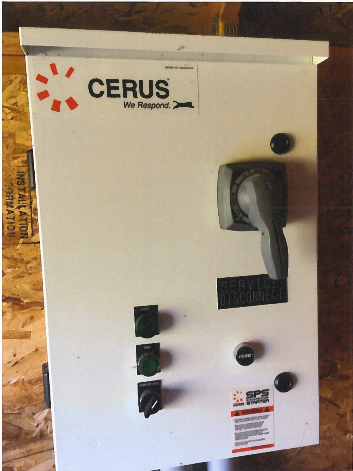
Irrigation pump control panel
