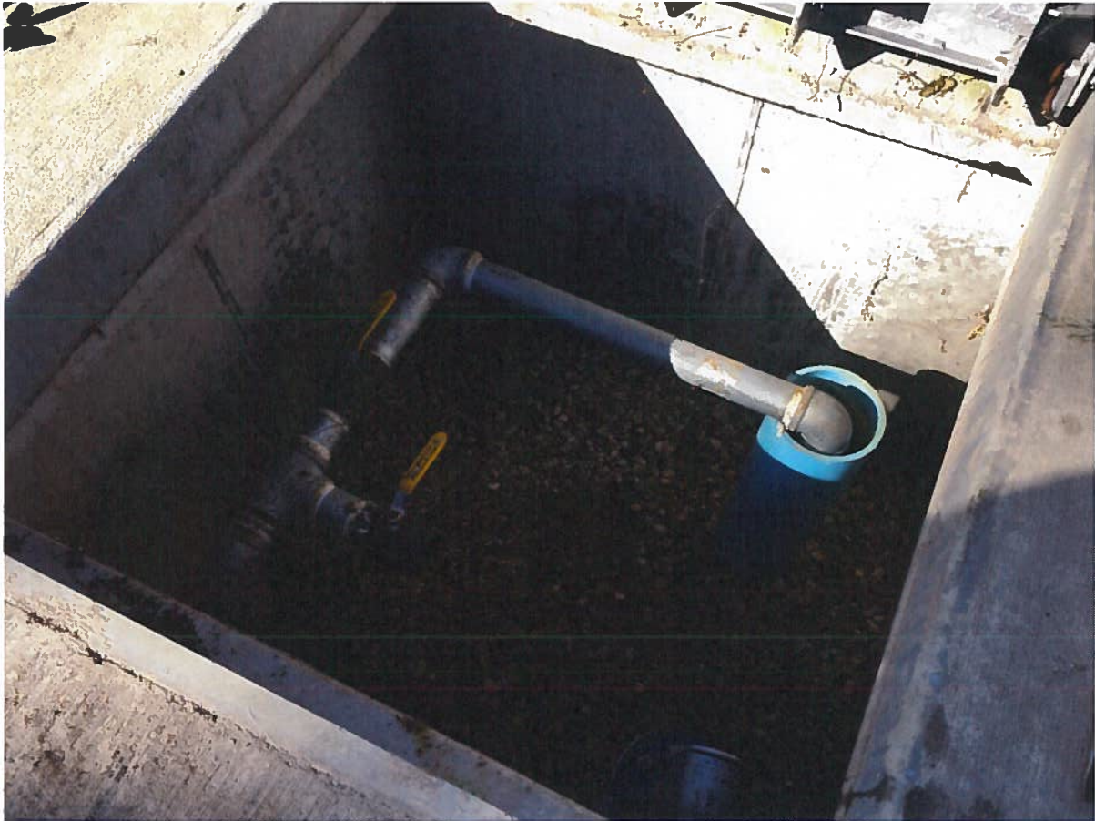
Vault with well discharge to pond fill pipe. Flow measurements taken by connecting to lower ball valve with yellow handle
