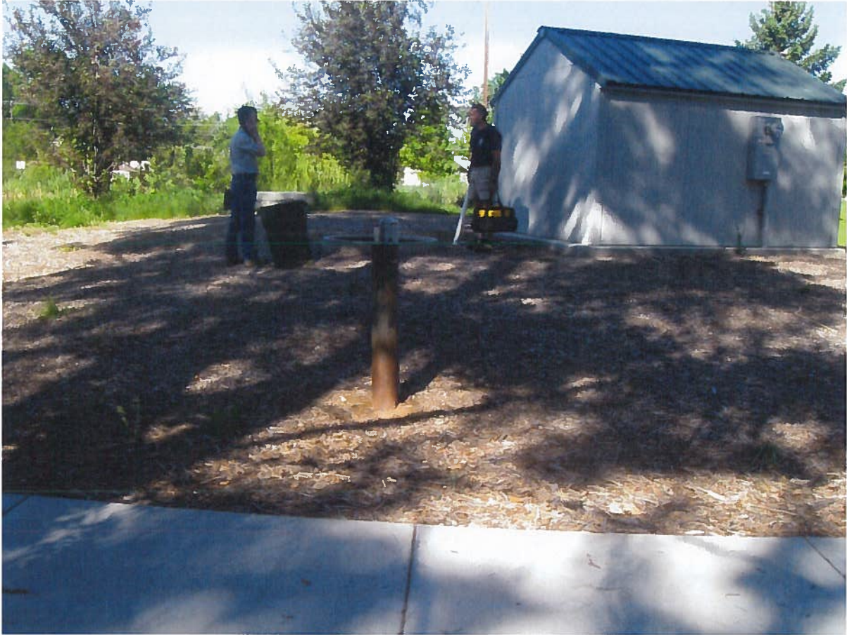
Well casing in foreground. Pump house in background.
