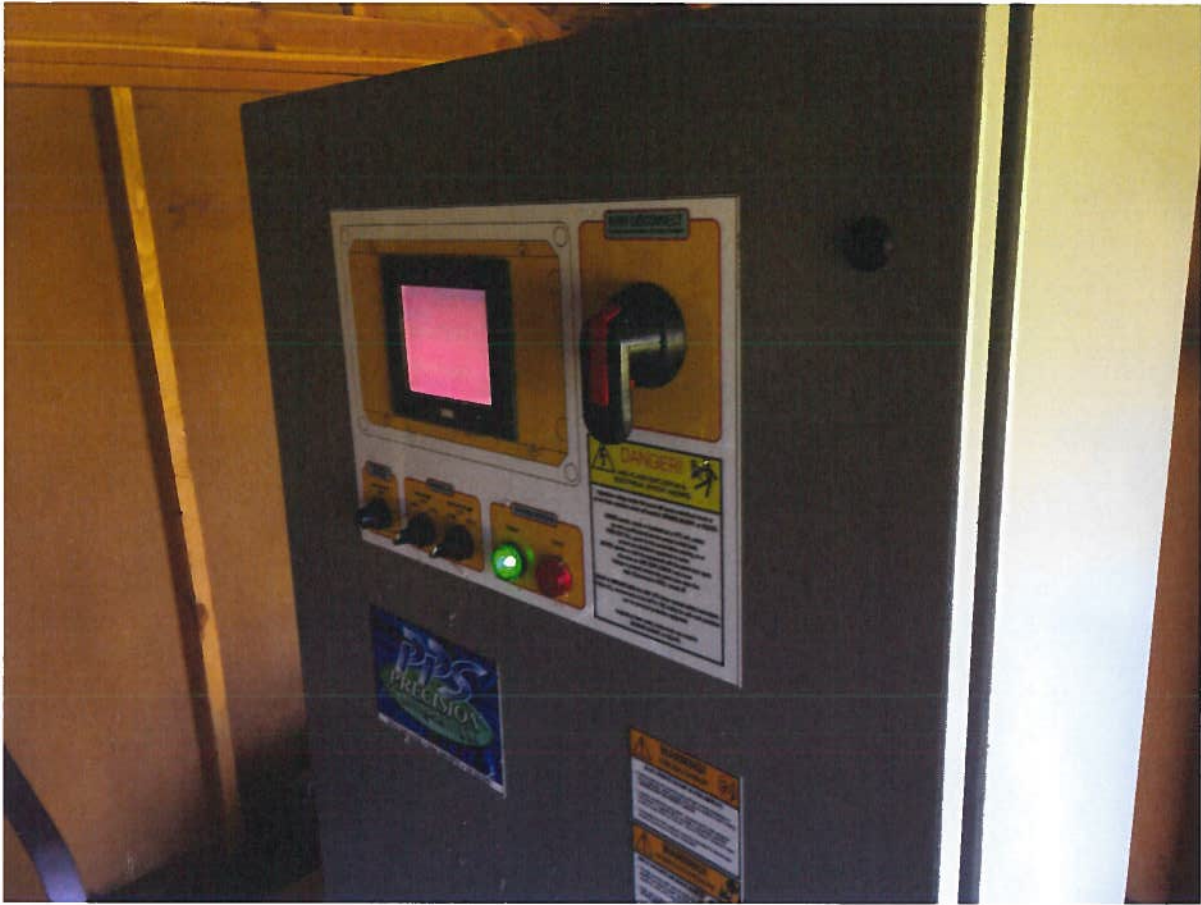
Pressure irrigation pumping system motor controls
