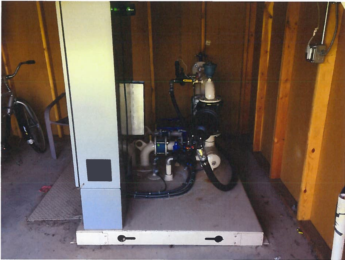
Pressure irrigation pump system pump skid. Submersible pumps in wet well below pump skid.
