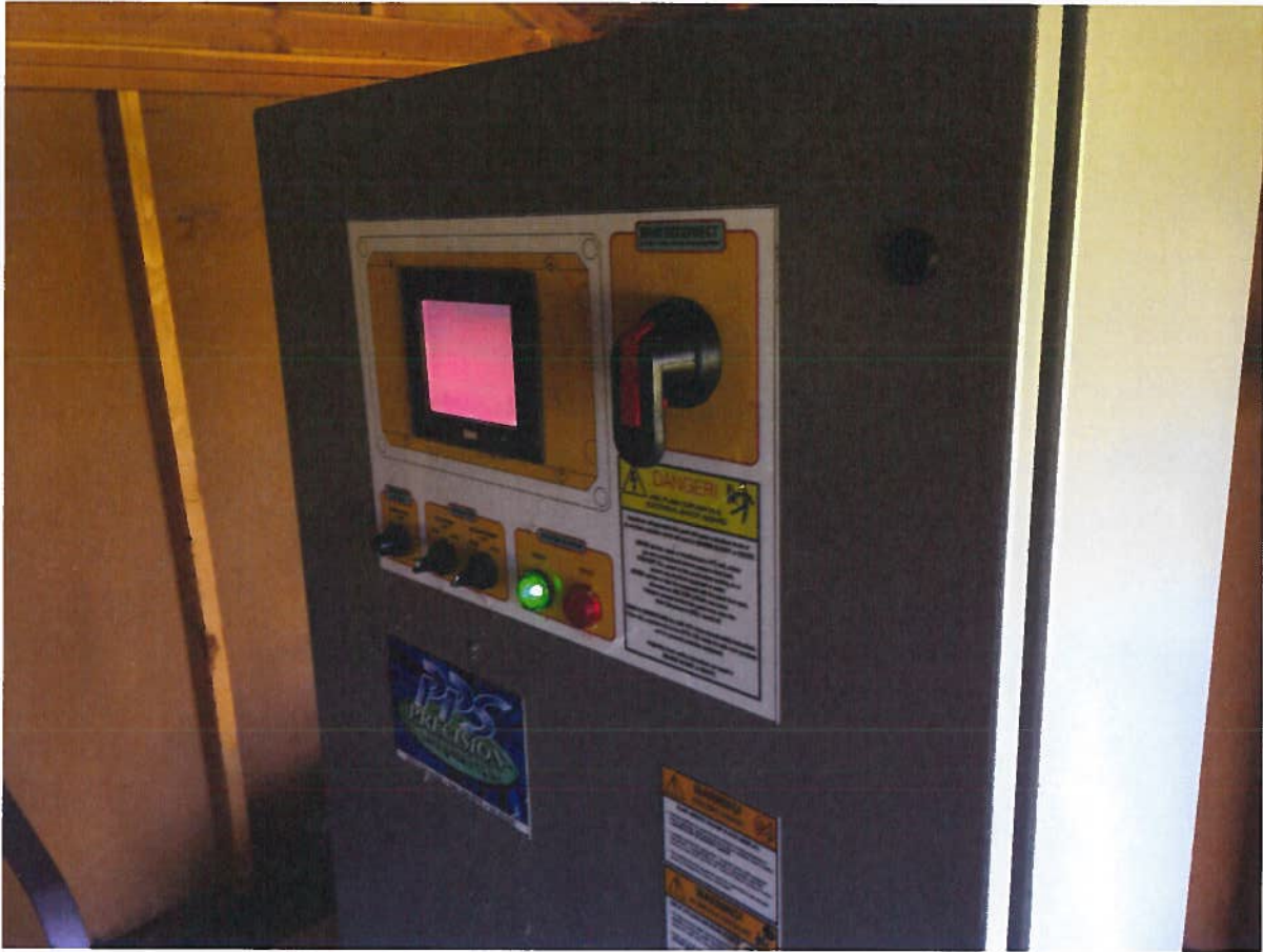
Pressure irrigation pumping system motor controls
