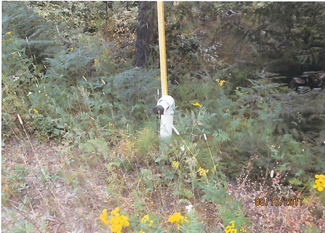
Dry hydrant to be used by fire department in case of fire.
