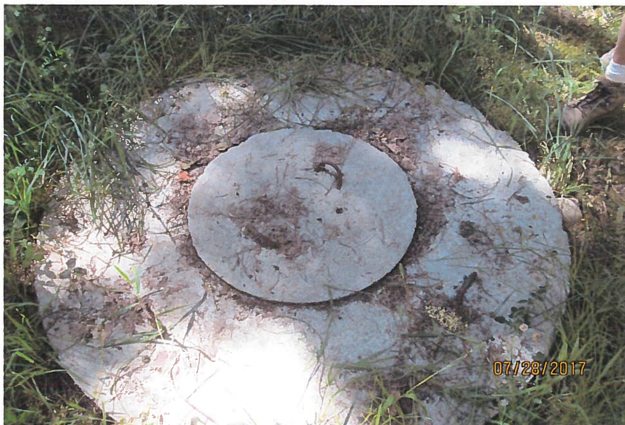
POD, hand dug well with pump set at 10 feet.
