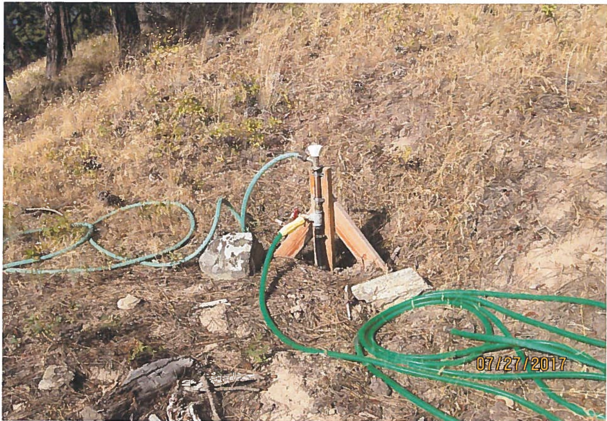
Frost free hydrant.
