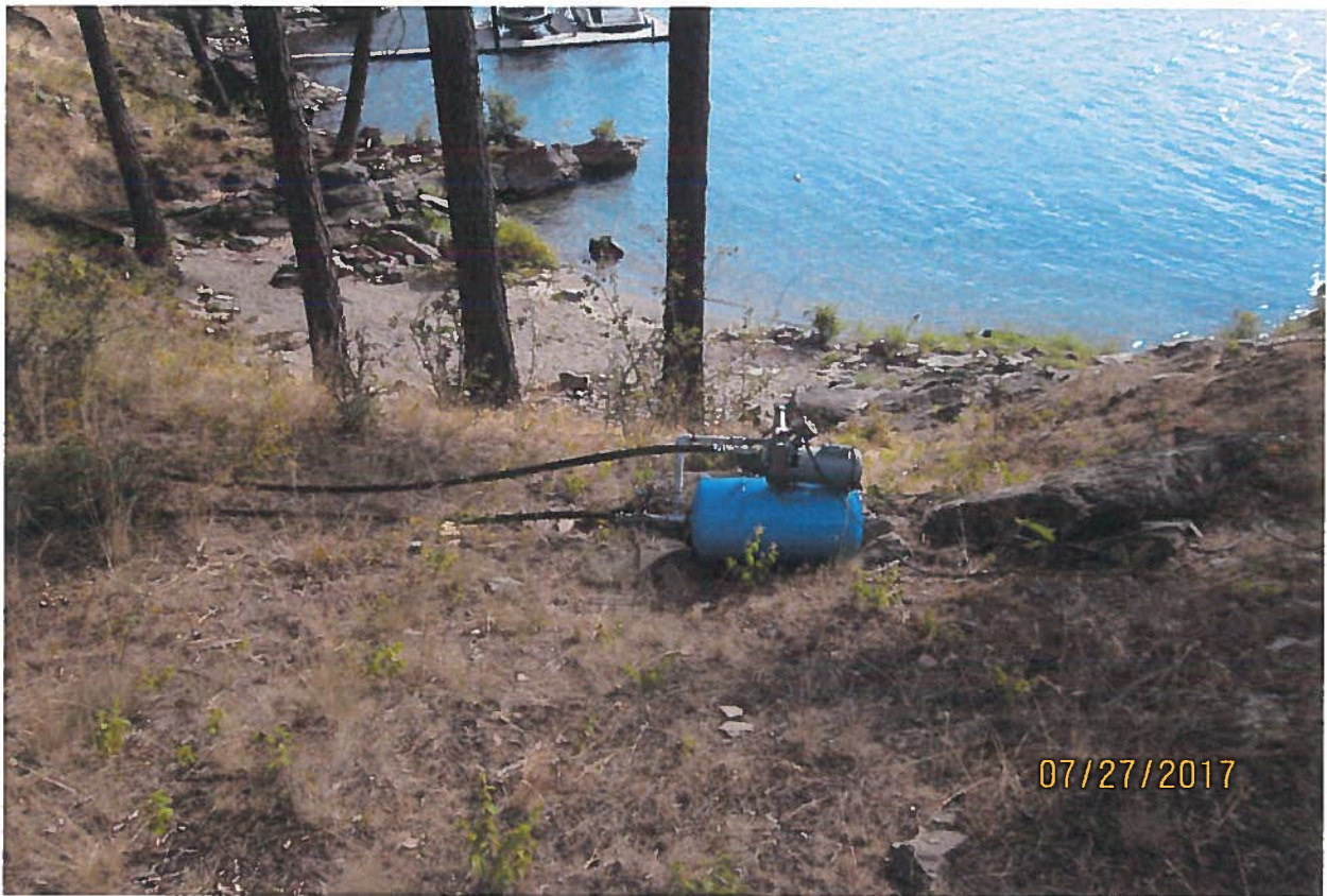
Pump with pressure tank.
