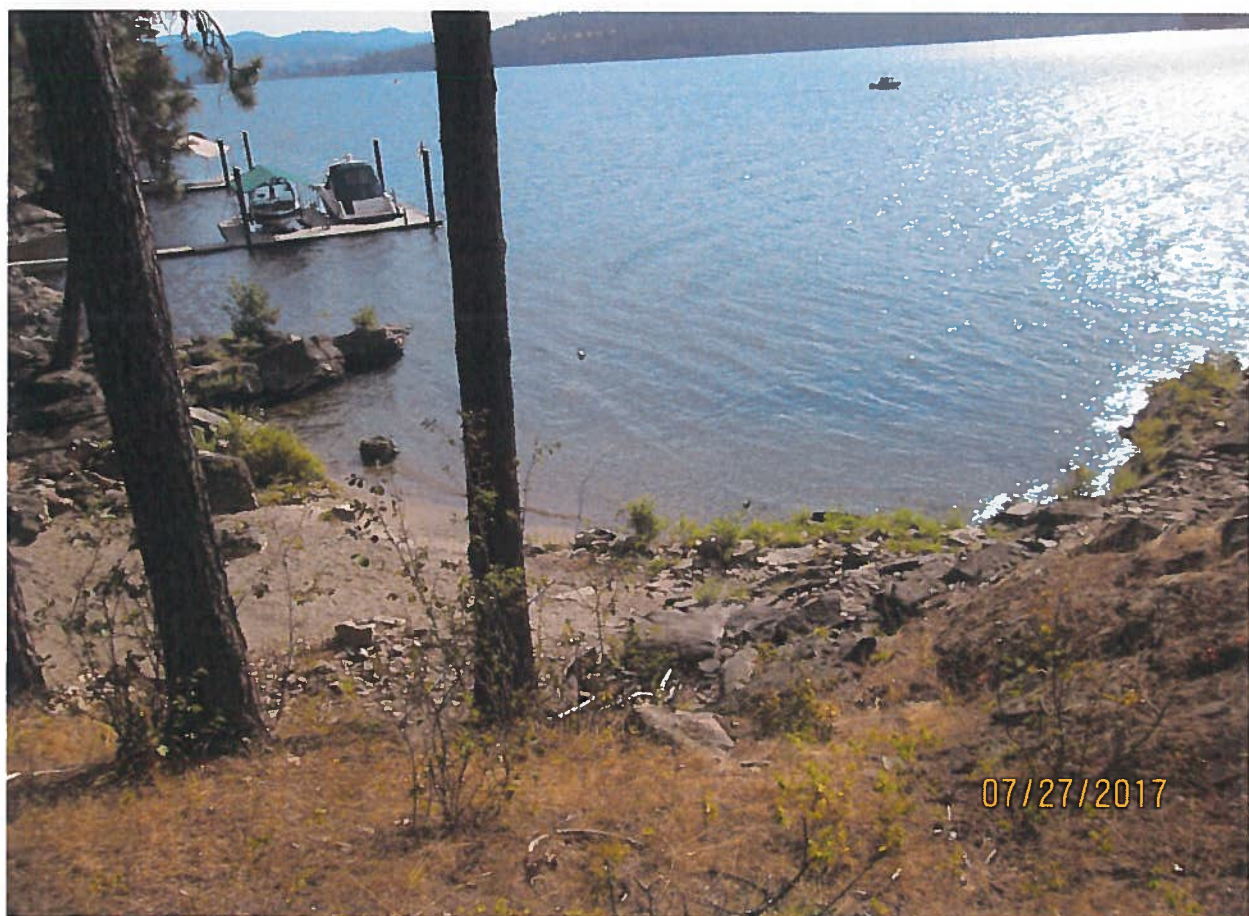
1 inch pipe going into lake with buoy marking location.
