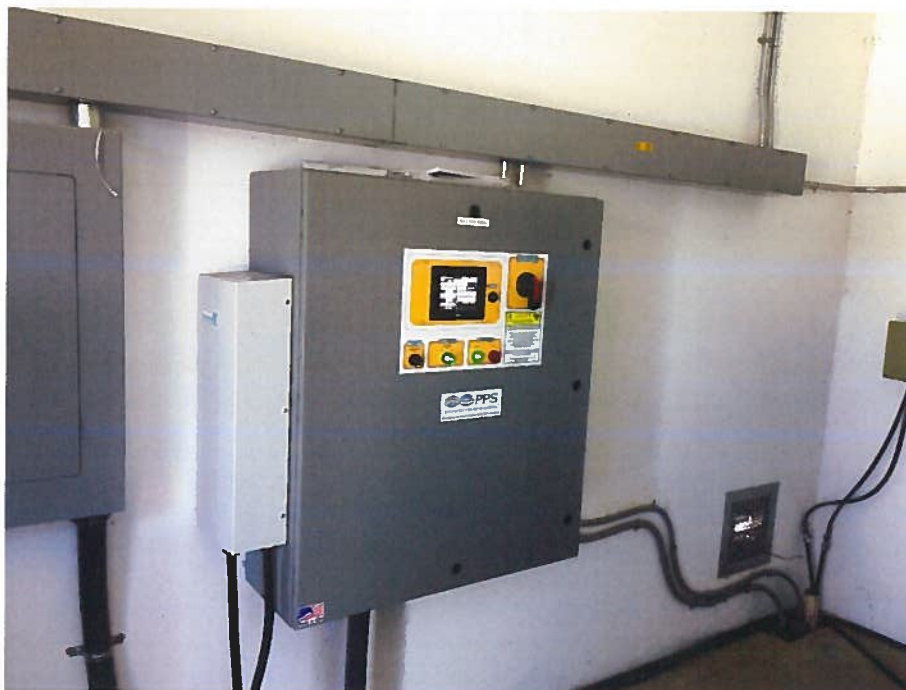
Pressure Irrigation Pumping System Motor Controls
