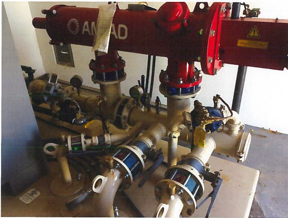
Surface Water Pump Station from Pond
