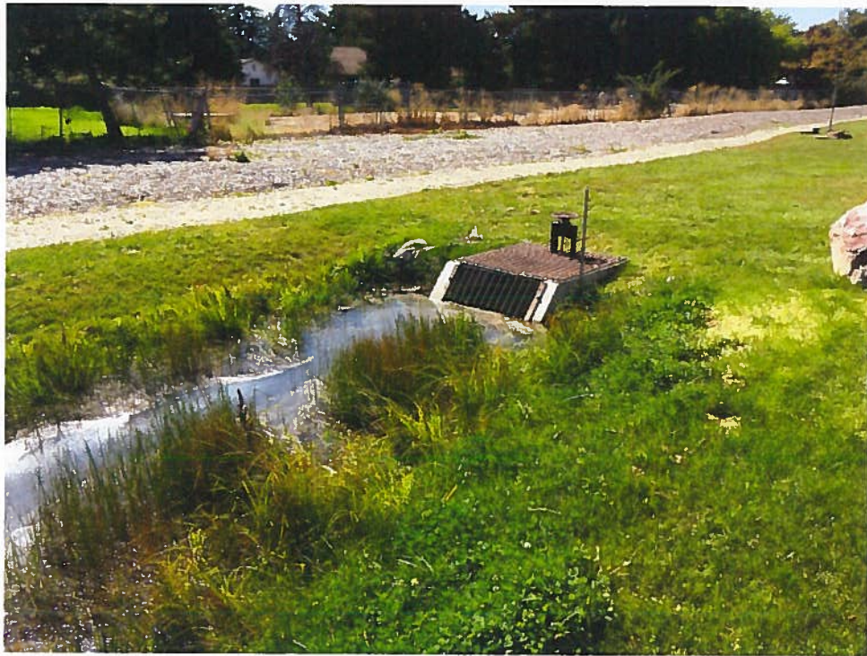
Surface Water Delivery Inlet to Pond
