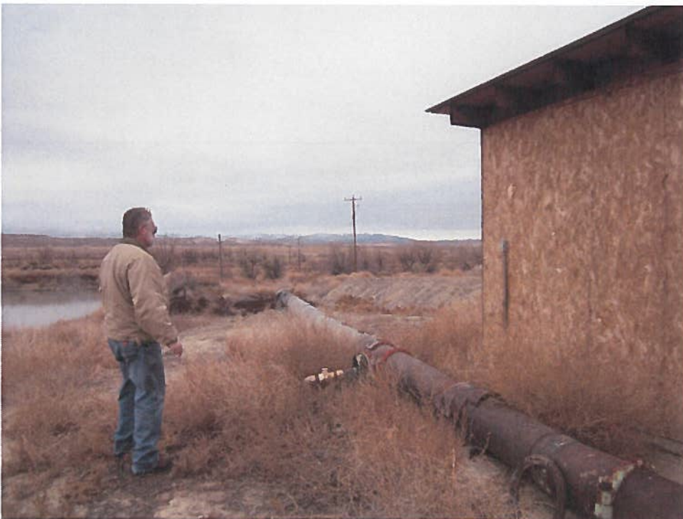
The pipe provides geothermal water for the heating system in the greenhouses. No pump is required for the heating system.
