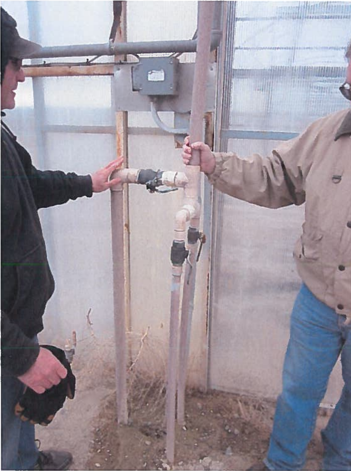
Controls inside the greenhouse
