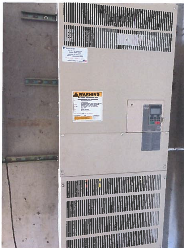
Well 3 VFD control panel
