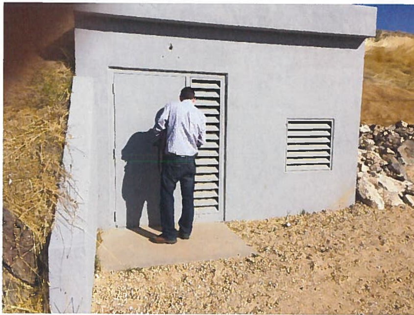
Well 3 well house
