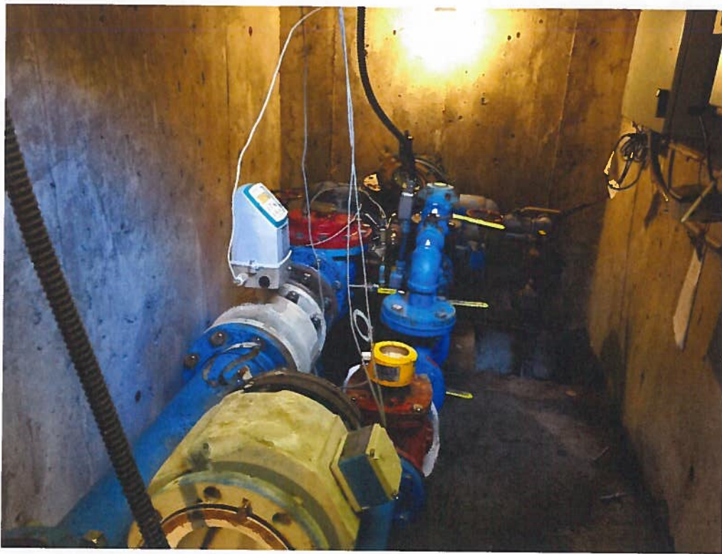
Discharge pipes and flow meters in River discharge monitoring station vault
