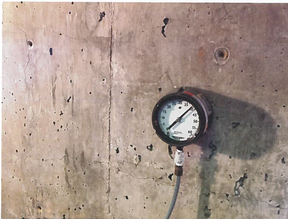
Pressure gauge in river discharge monitoring vault
