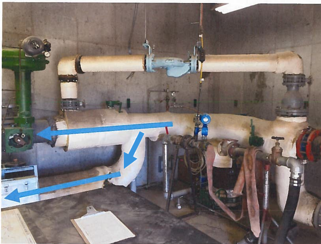
Well 2 well house mechanical piping; blue arrows show direction of flow.
