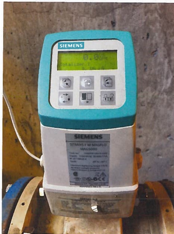
High flow Siemens mag meter for river discharge
