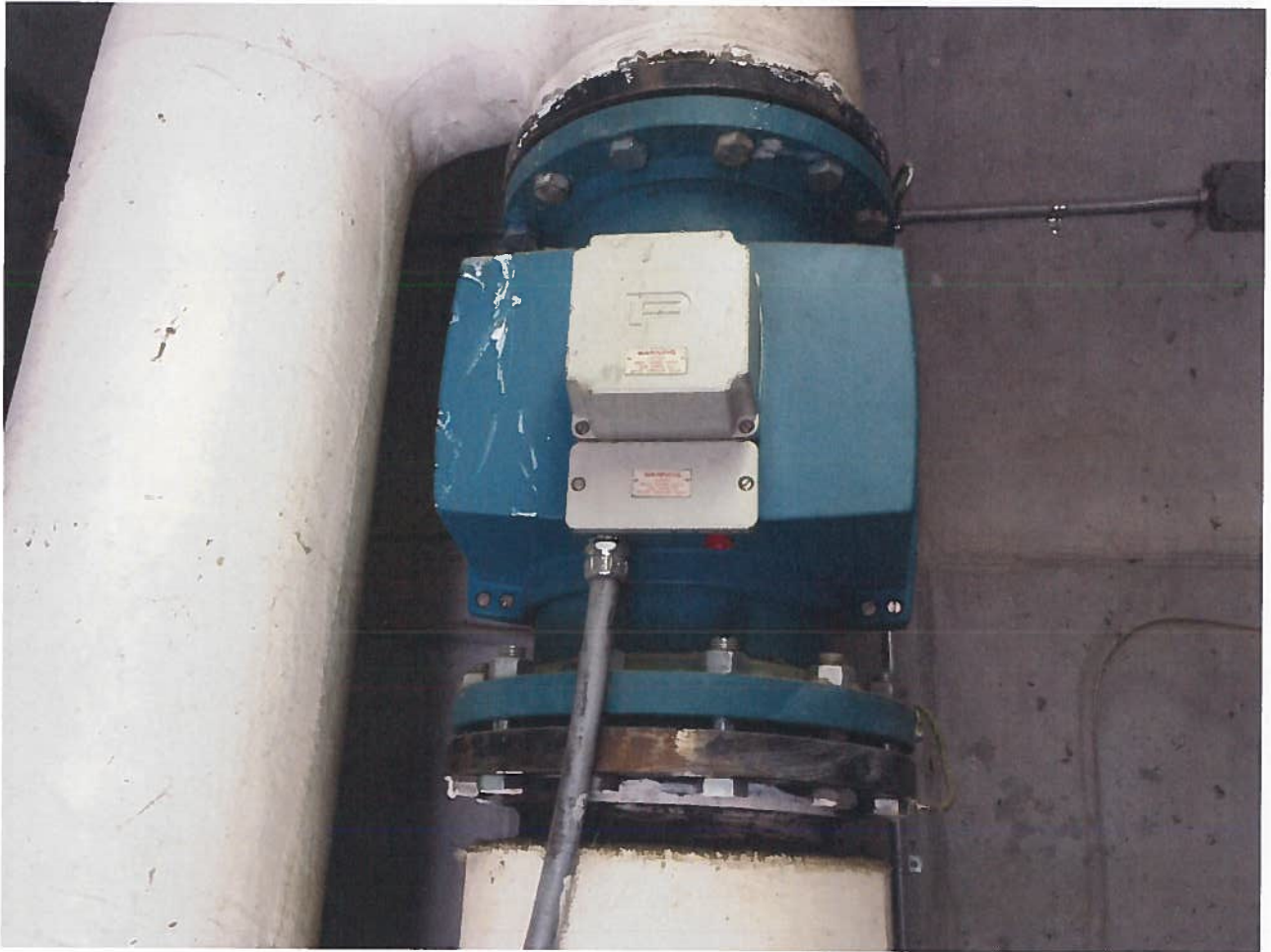
Fischer Porter flow meter. Flow meter in the Well 2 well house measures the combined flow from Wells 2, 3, and 4.
