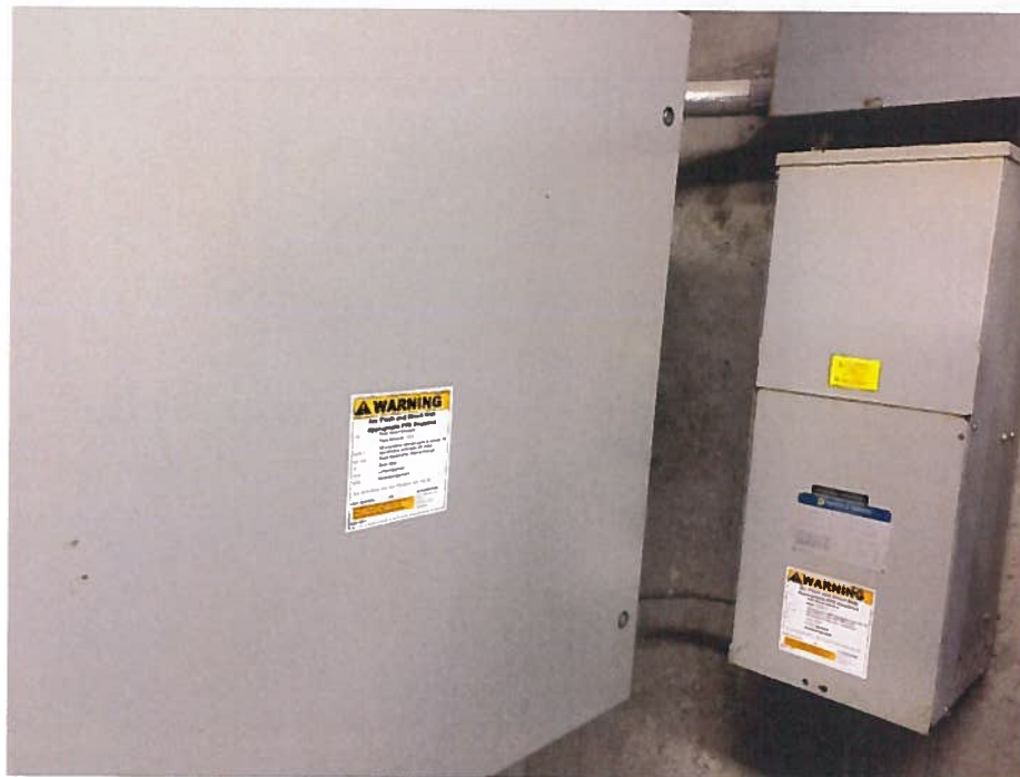
Well 4 VFD control panel
