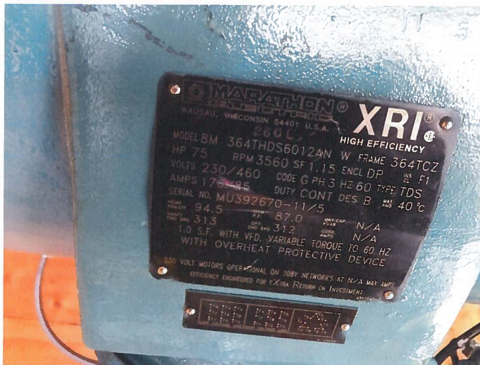
Injection booster pump name plate
