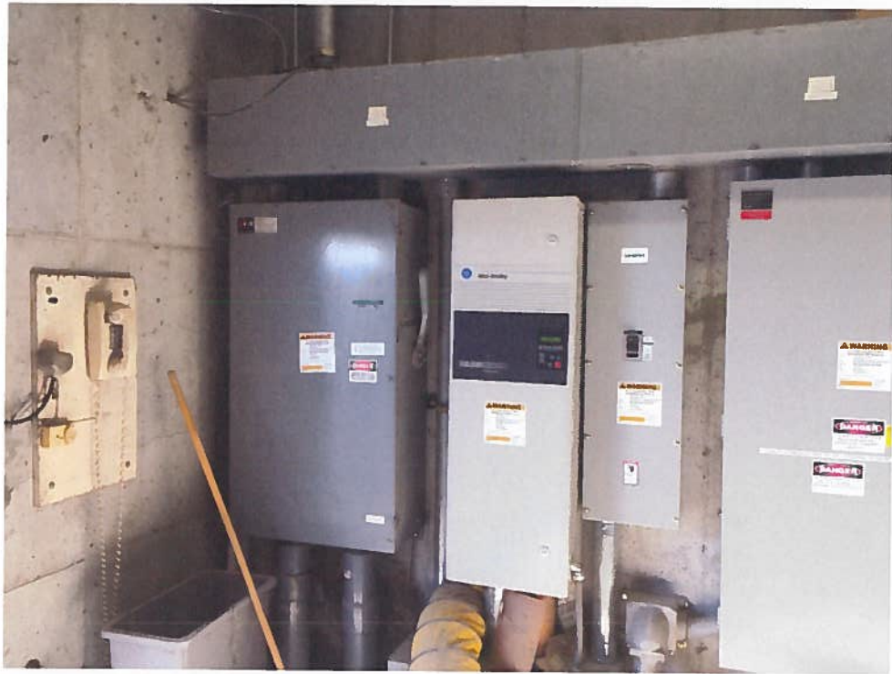
Well 2 pump VFD control panel
