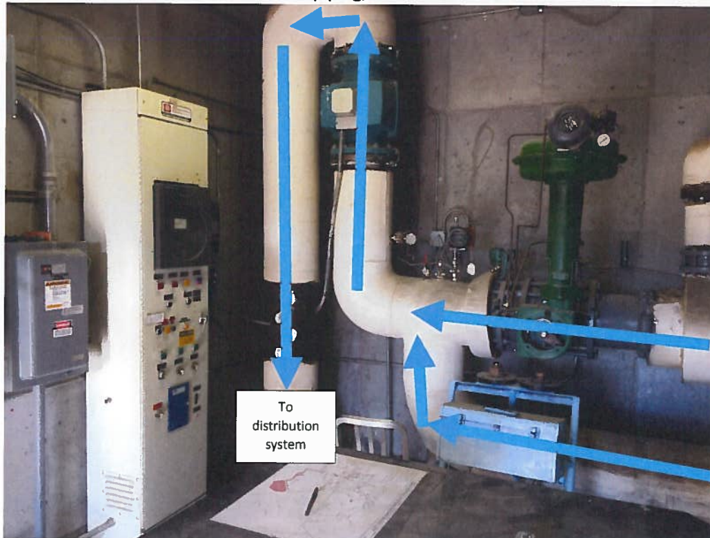
Well 2 well house mechanical piping; blue arrows show direction of flow.
