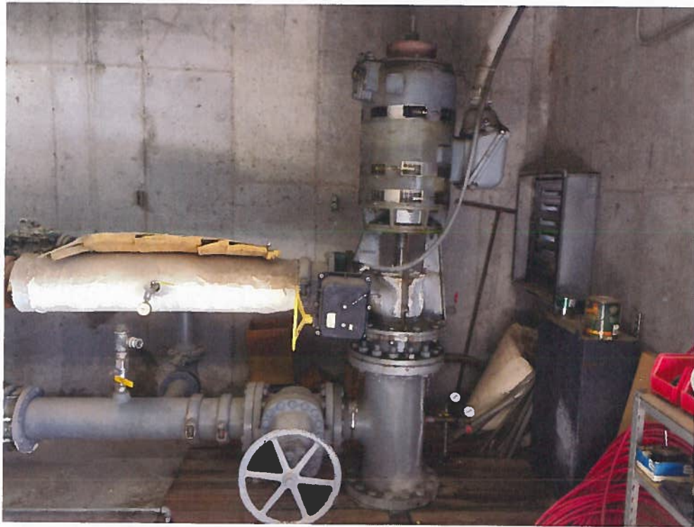
Production Well 2 with 125-hp vertical turbine pump
