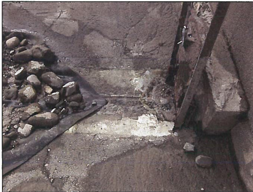
Figure 2: Lower spring unmeasured flow estimated at 5 gpm.
