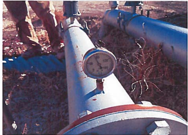
North Line Pressure Reading
