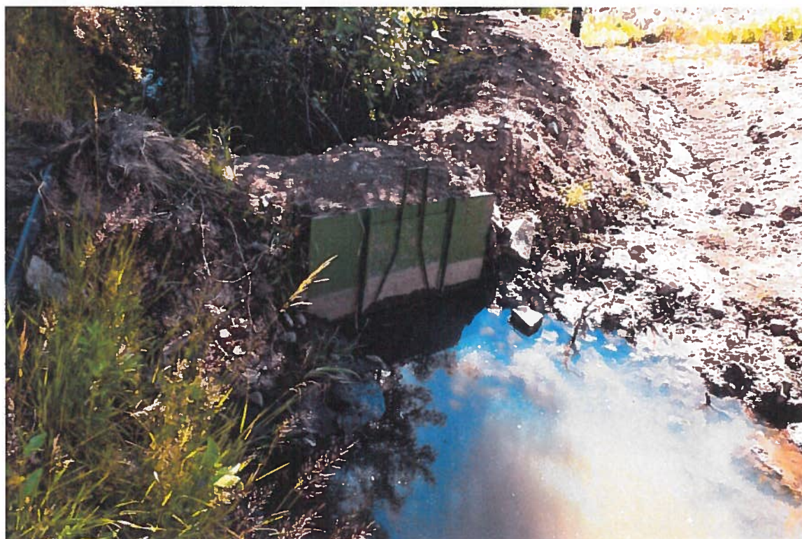
Lockable headgate above the spring collection pipe with overflow bypass for heavy runoff.
