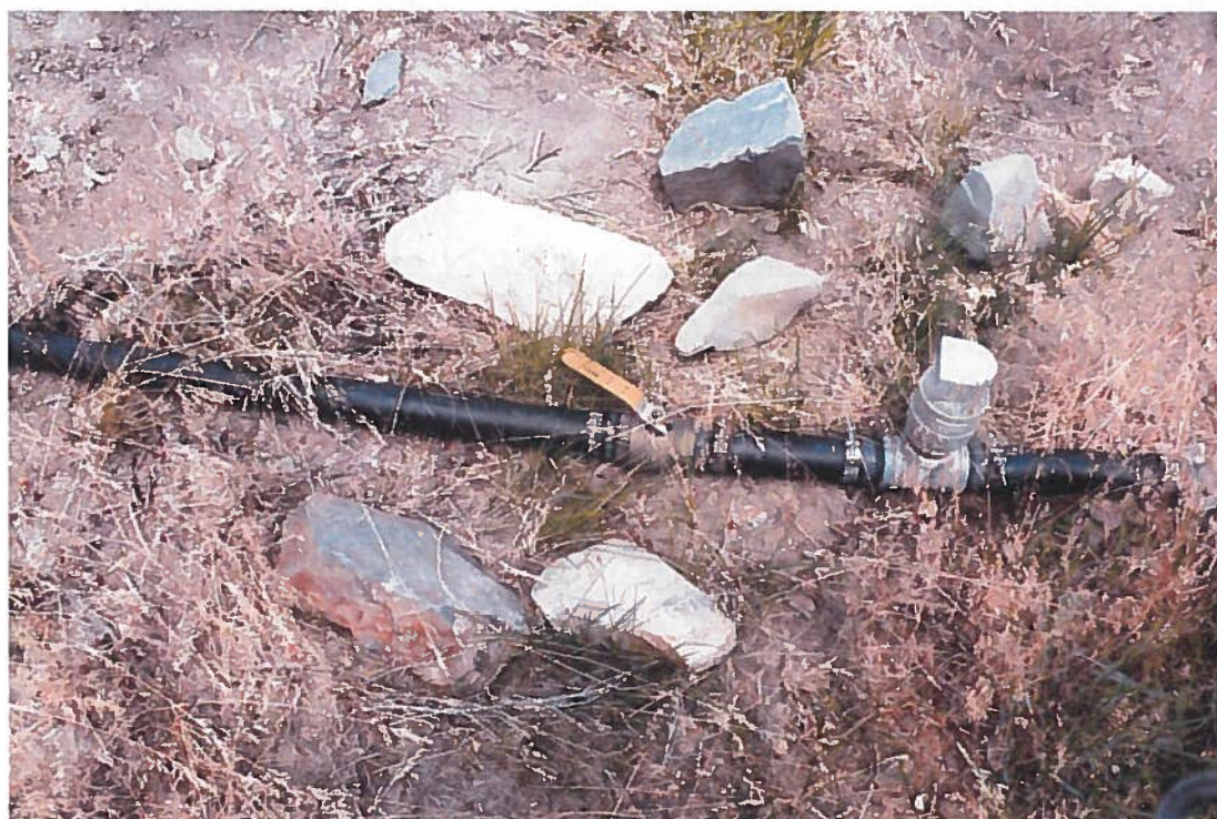
Air release and shut off valve from the spring collector to the bottom of the hill
