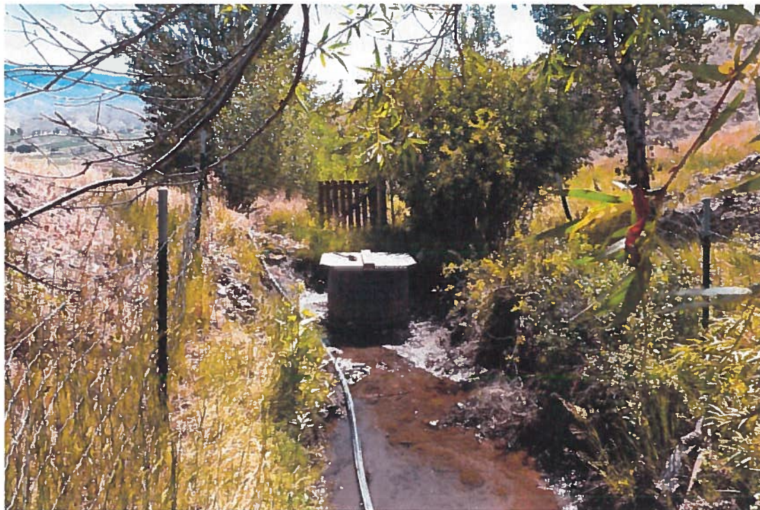
Spring water collection pipe: A 2 inch pipe runs down to the bottom of the hill for irrigation.
