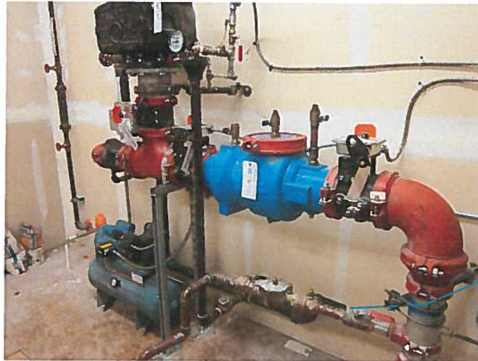
Two inch copper supply line
