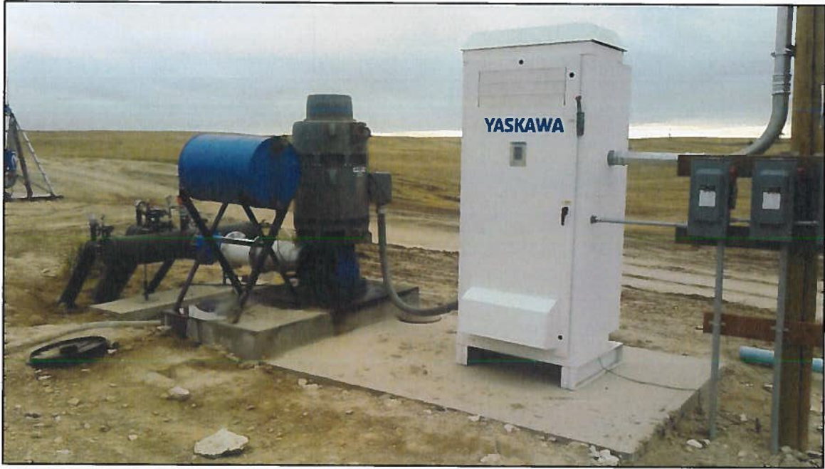
Figure 1: Well #1 (Section 17) is 200-hp vertical turbine.
