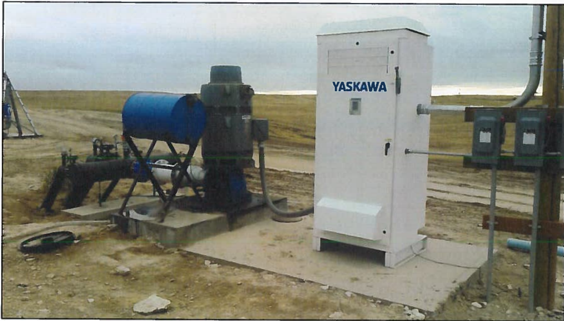
Figure 1: Well #1 (Section 17) is 200-hp vertical turbine.
