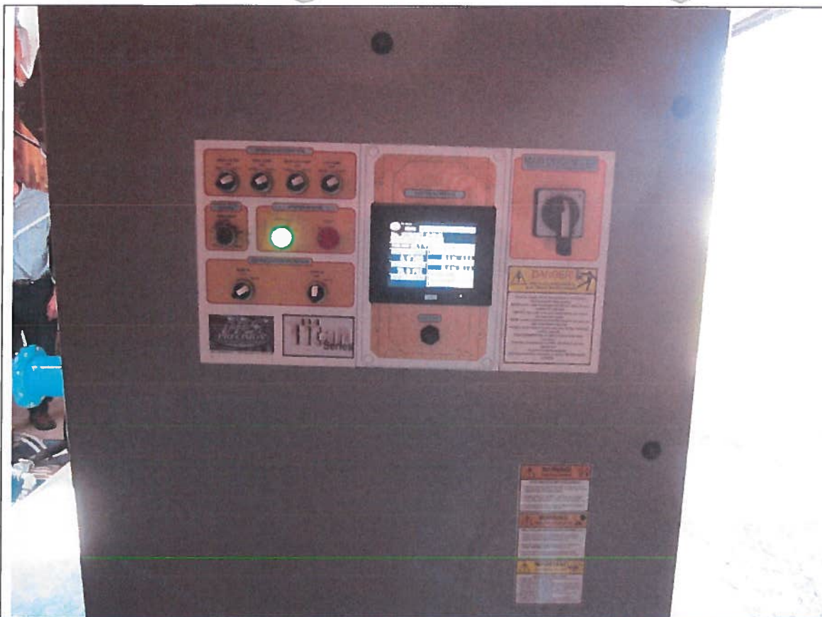
Control panel for the recirculation and irrigation system.
