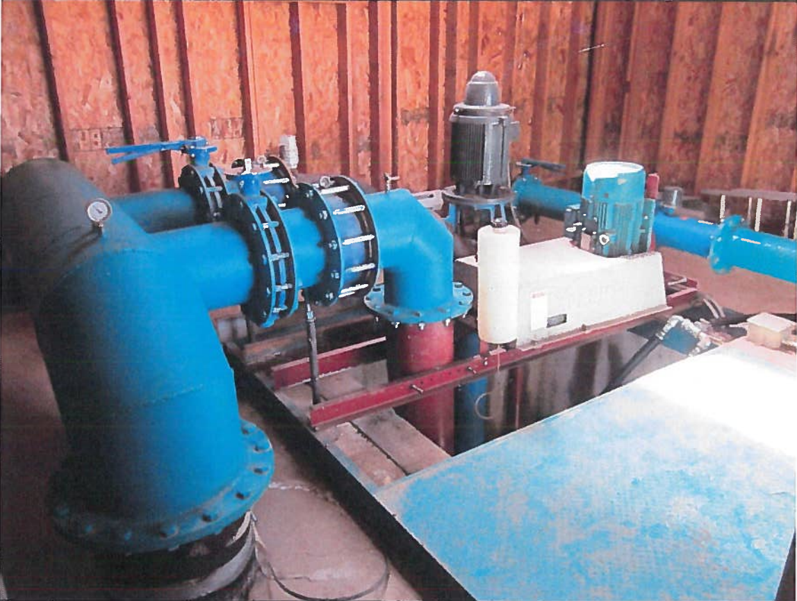
Recirculation pumps inside the pump station.
