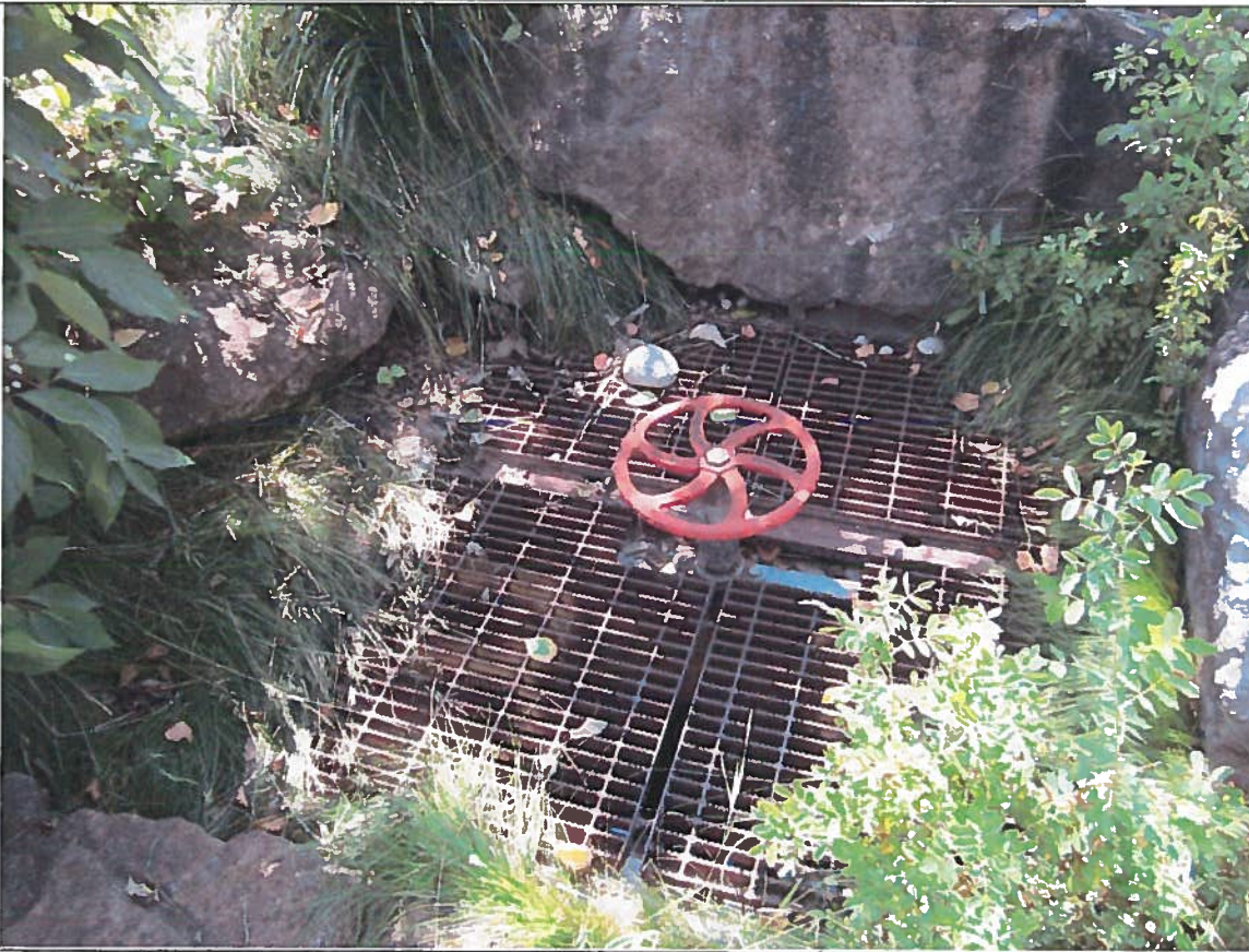
Control gate for Pond 2B. East side of S. Bellemonte Way; in between Watersford Drive and Sherington Drive.
