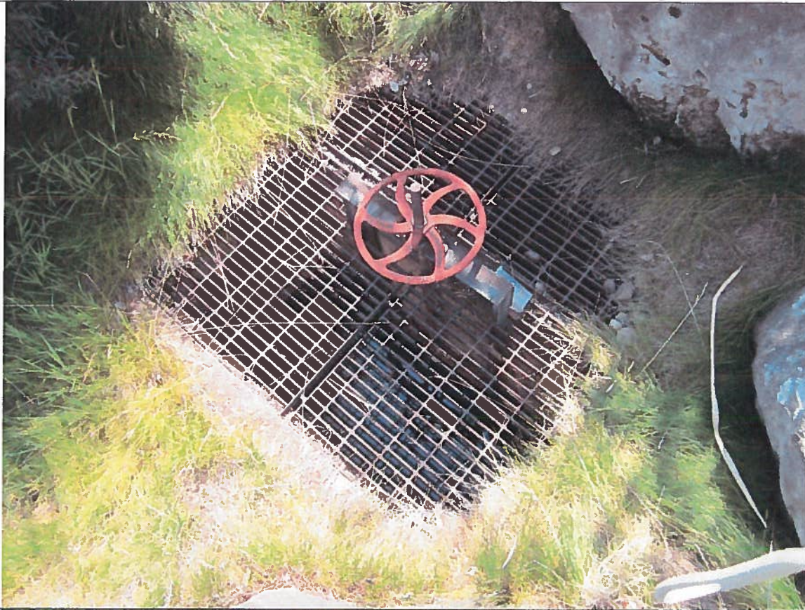
Control valve for Pond 1B. Located on the east side of S. Bellemonte Way.
