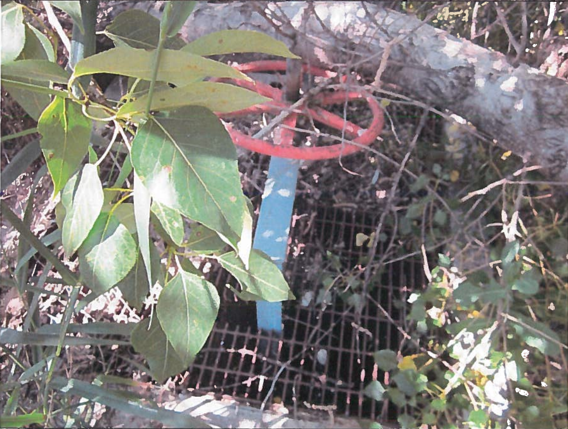
Control Valve located on the north end of Pond 5.
