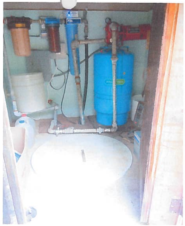
Pump House with 1 Hp pump, pressure tank, filters and UV light for water purification; Cement 1000 gallon holding tank
