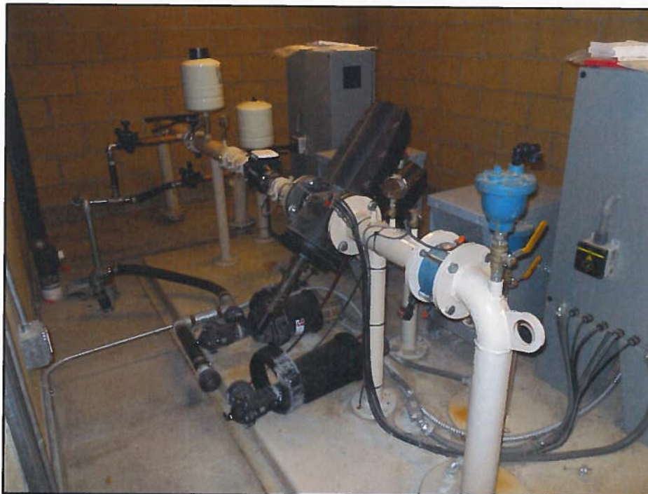
Figure 8. Irrigation control room
