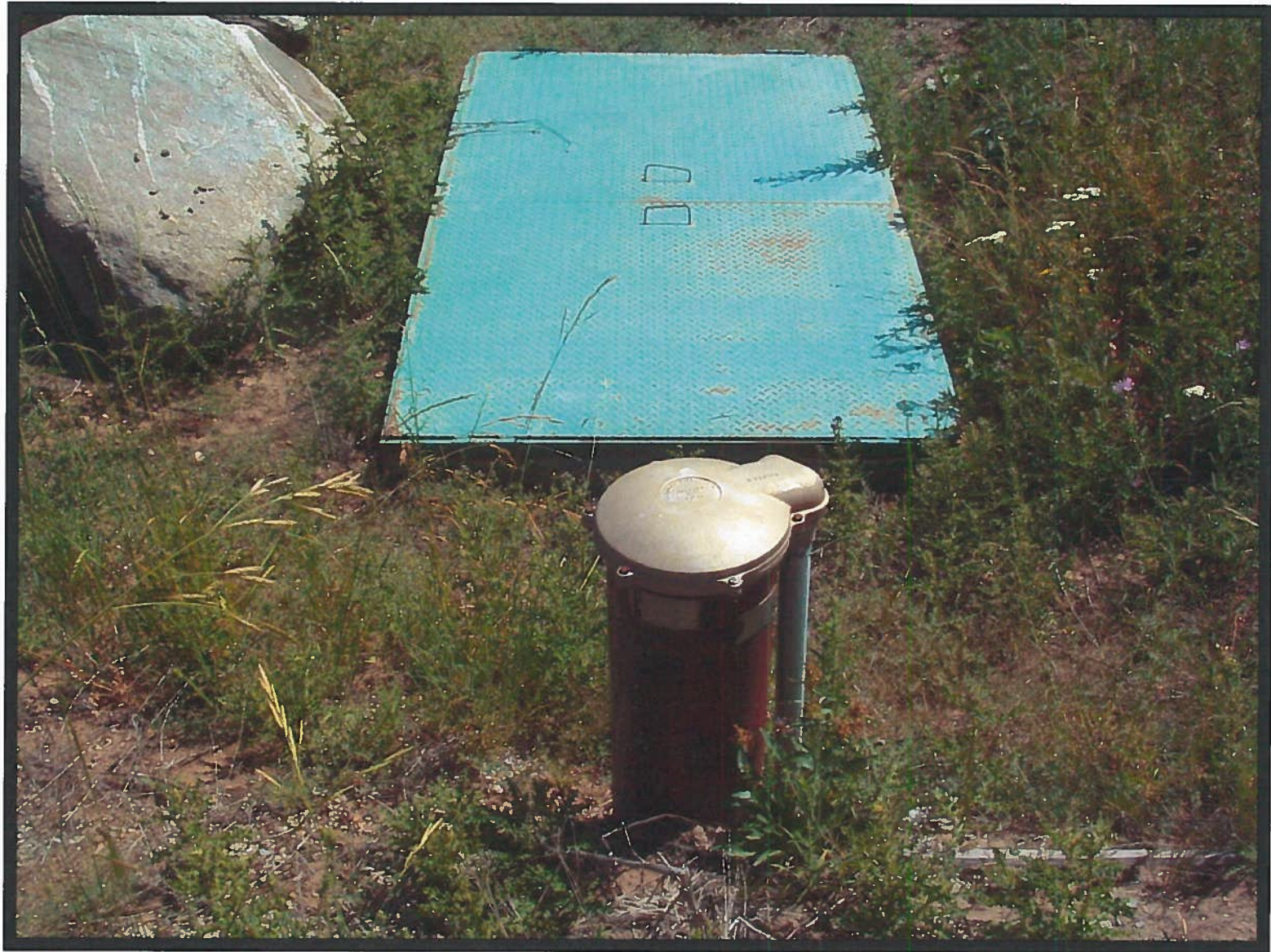
Well 2 and Flowmeter Vault
