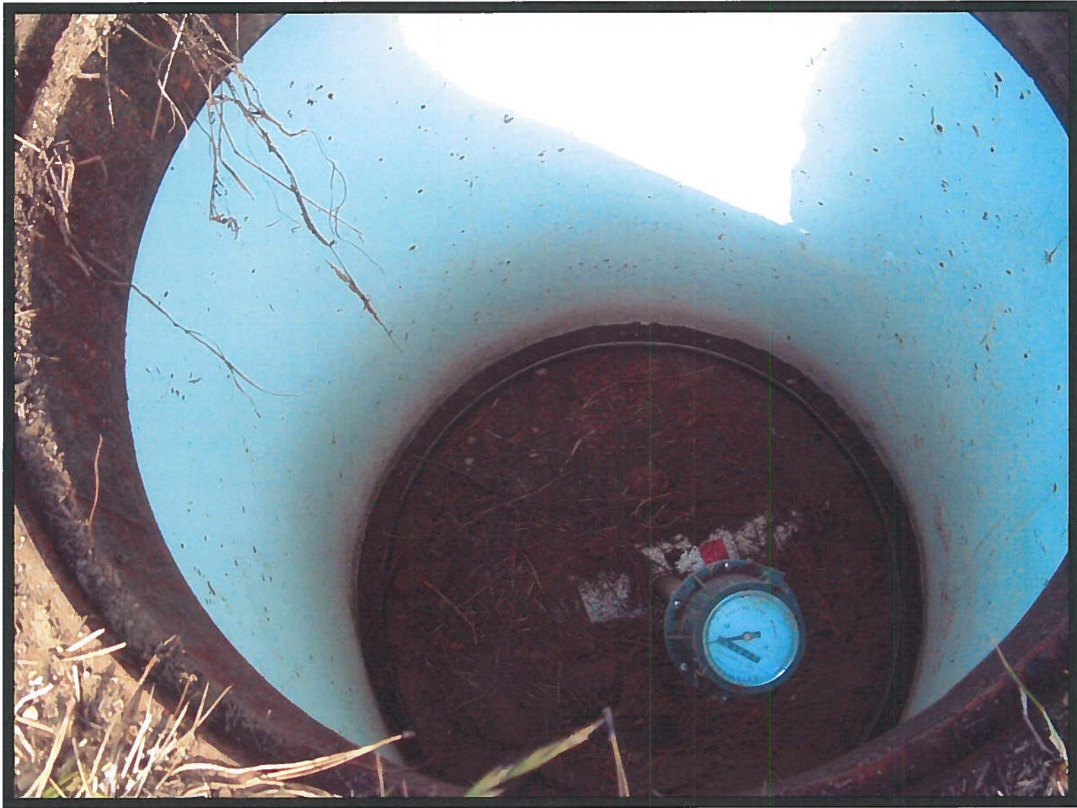
Payette Lake Pump Flowmeter
