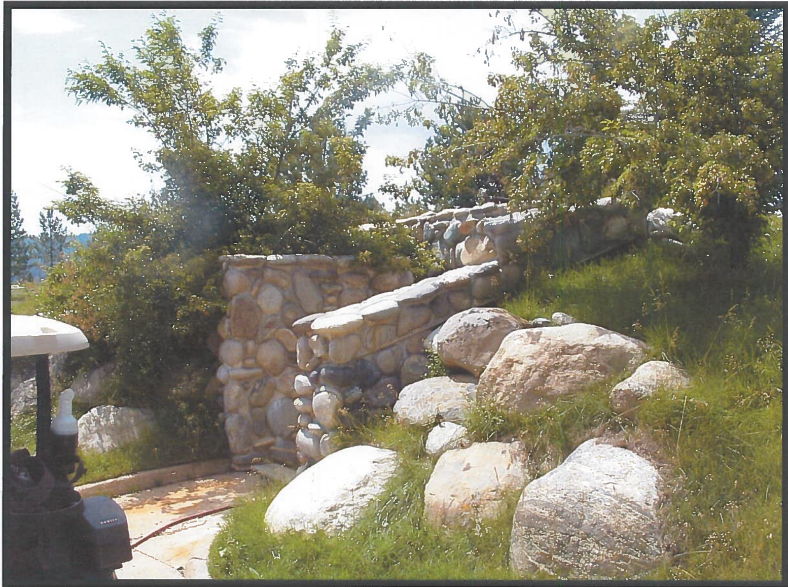
Pressure Irrigation Pump Station
