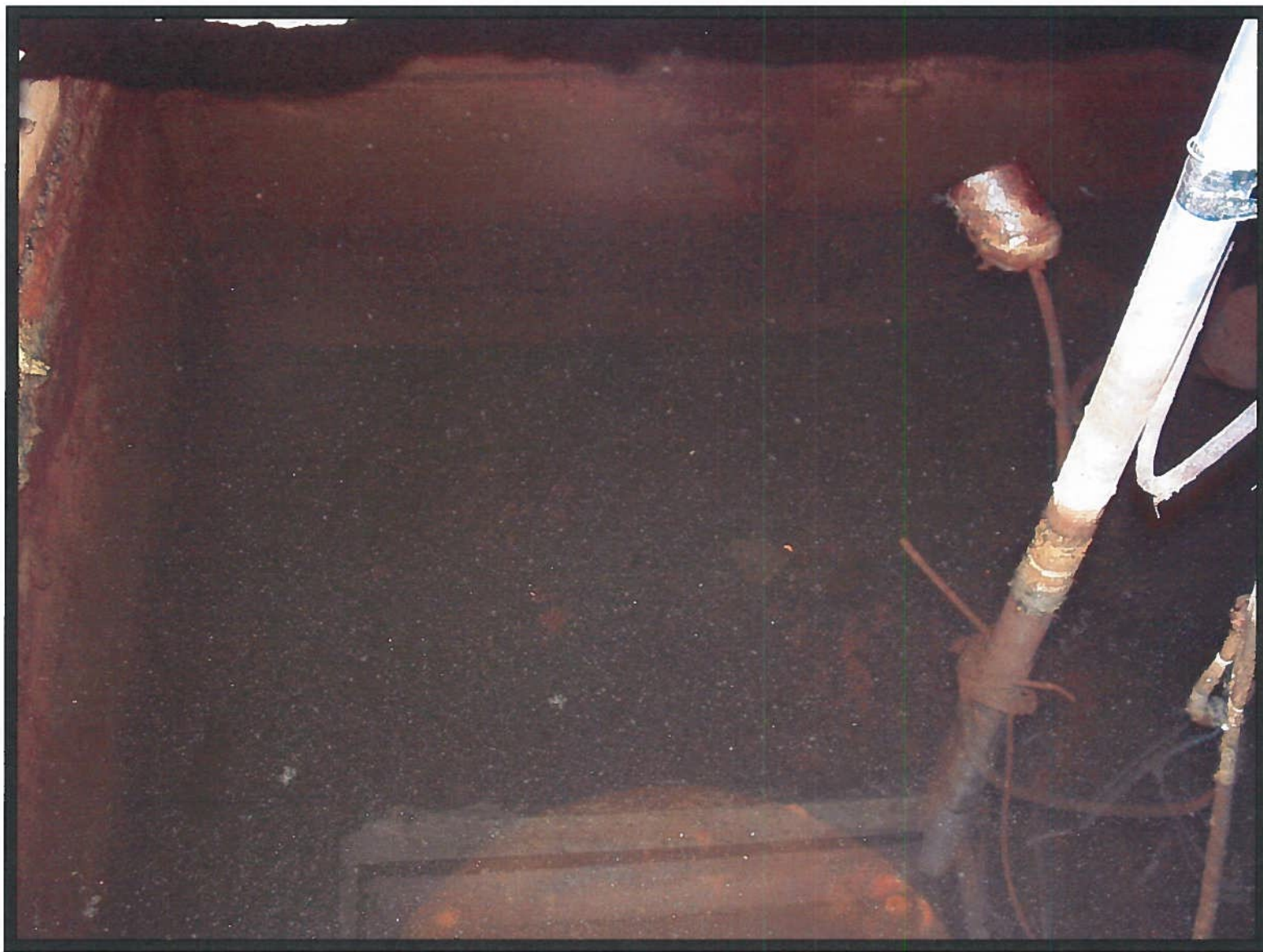
Looking Inside Pump Vault
