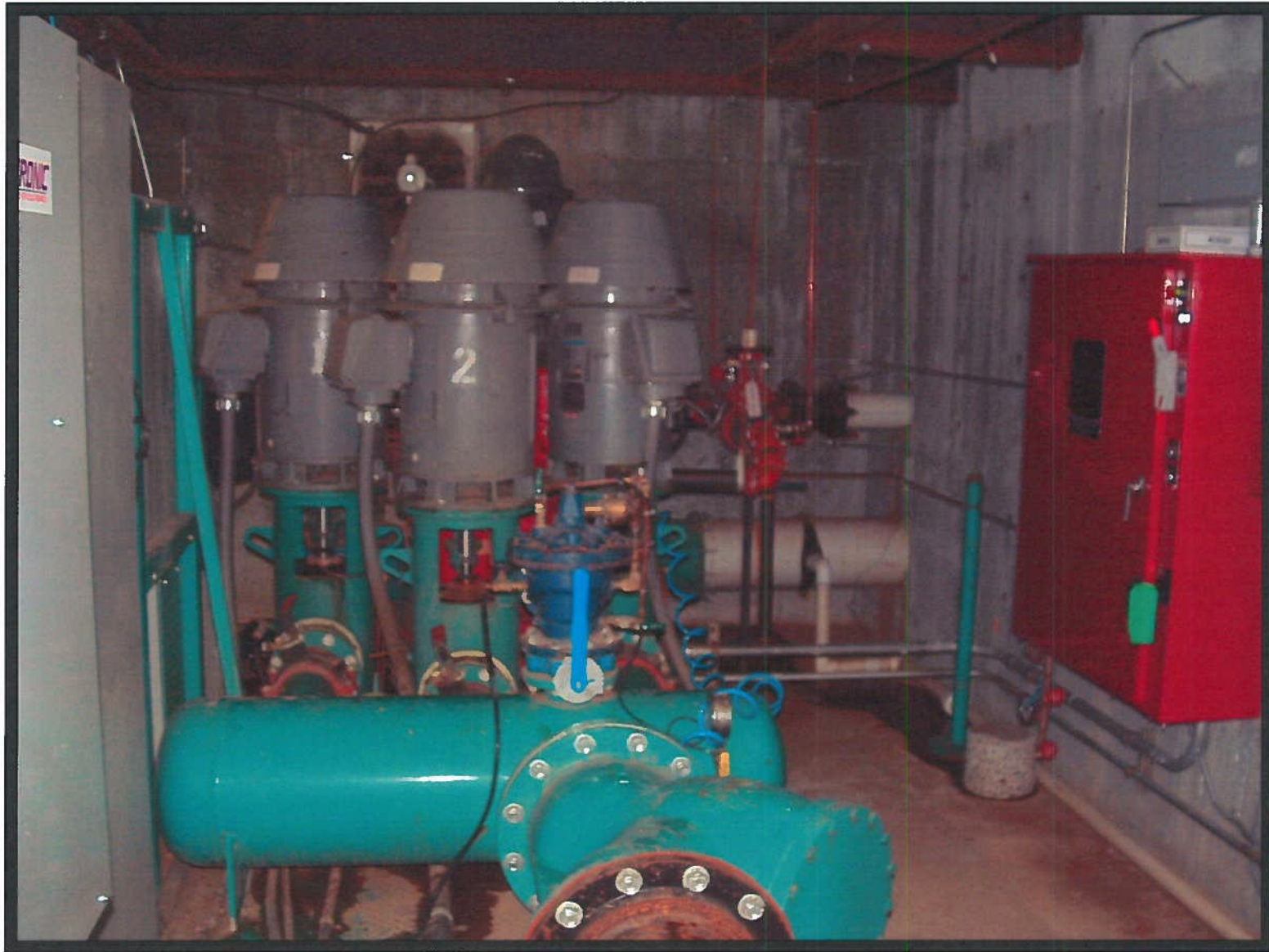
Three Irrigation Pumps at Whitetail Pump Station
