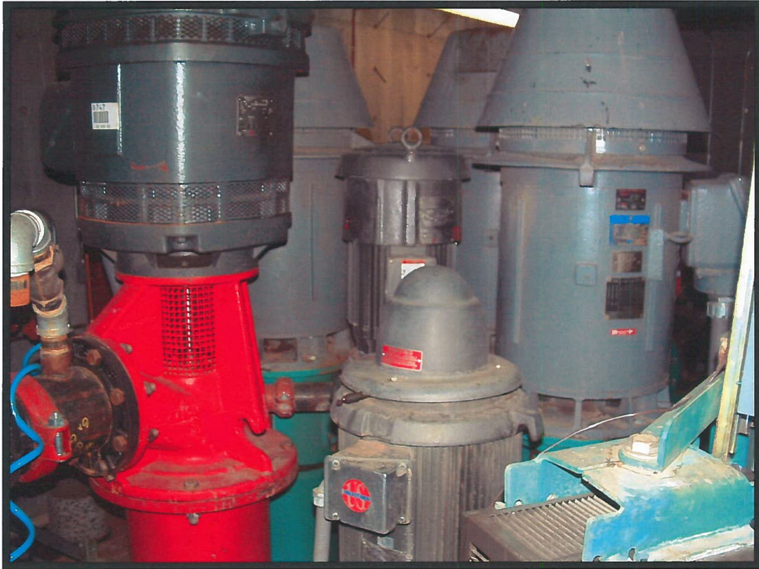
Whitetail Pump Station Pumps: 3 Irrigation, 2 Fire Protection and 1 Recirculation
