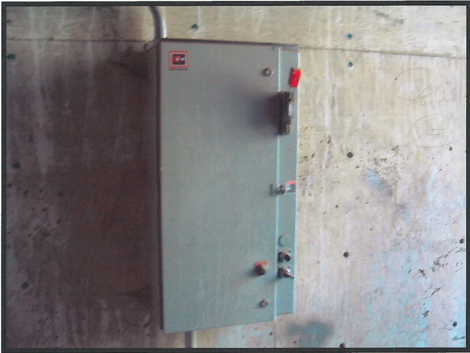
Lockable Pump Motor Controls
