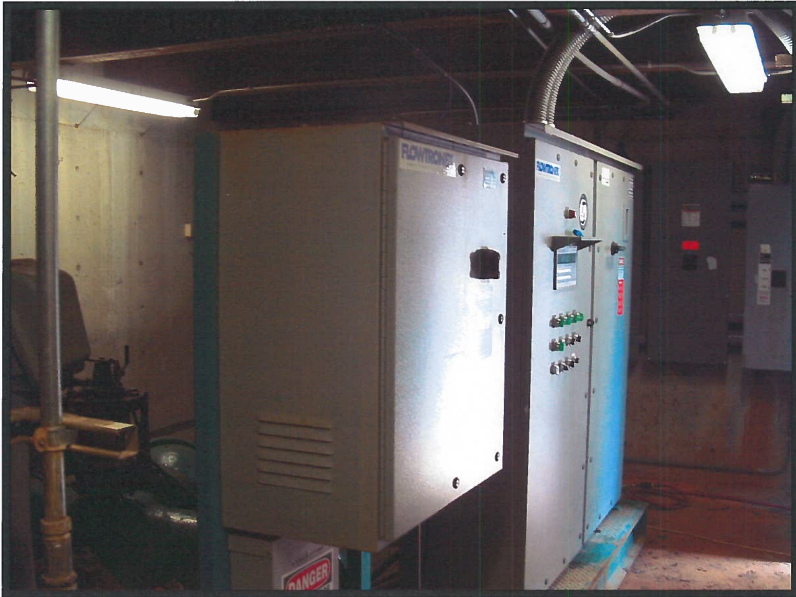
Whitetail Pump Station Motor Controls
