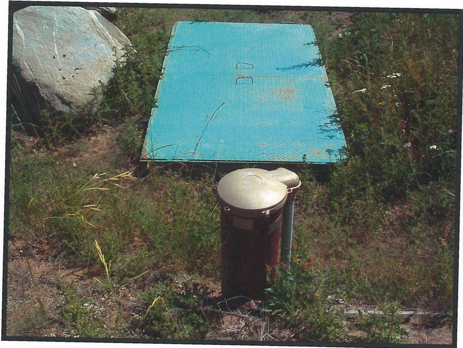
Well 2 and Flowmeter Vault
