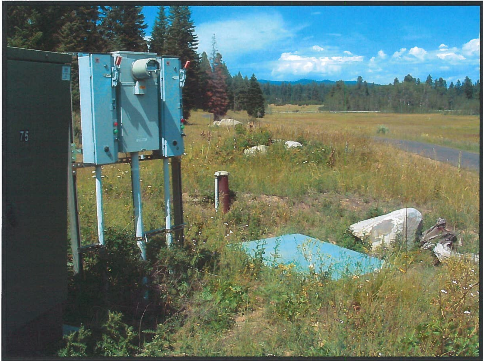
Well 7, Flowmeter Vault and Pump Motor Controls for Well 7 & 2
