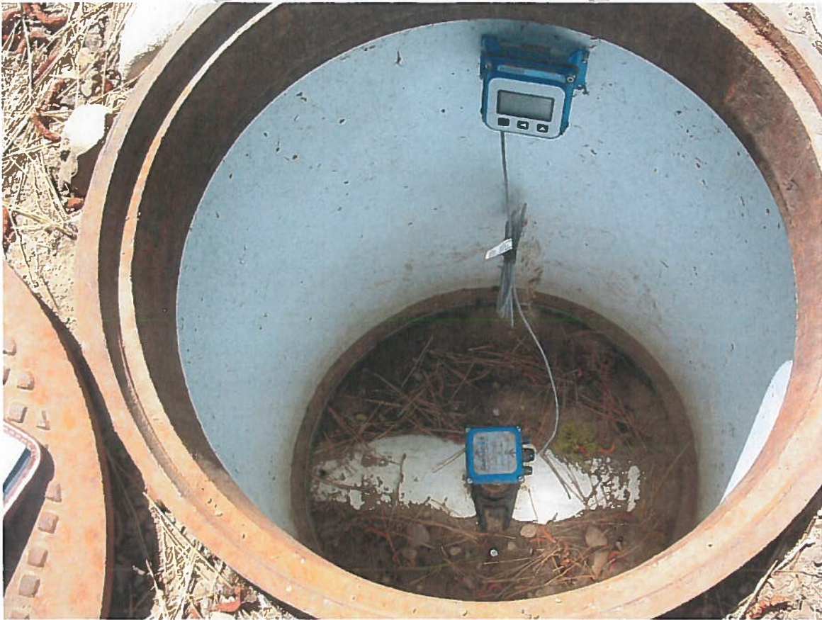
Figure 3 – Flow meter saddle-mounted to pipe and digital display.
