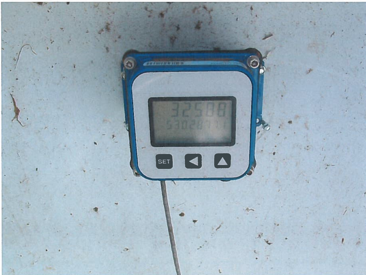
Figure 4 - Flow meter display. Upper number is instantaneous flow in gph. Lower number is total flow in gallons.
