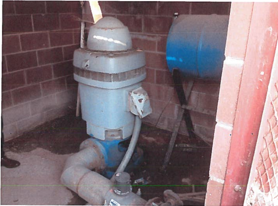
Figure 1 Well located in the pump house near the entrance of the subdivision. Water is diverted from the well using a 100-hp pump to an 8" pvc line.
