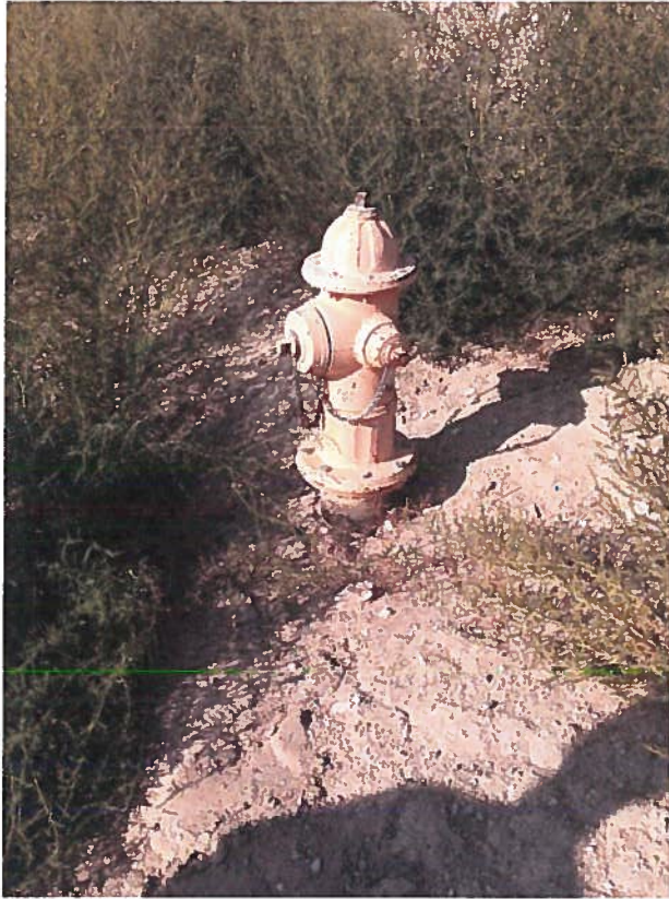
Figure 7 1 of the 3 fire hydrants used for fire protection in phase 1 of the subdivision
