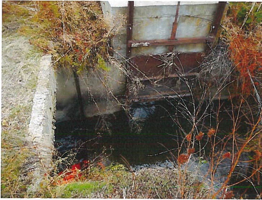
Photo 4. Gate to control the amount of water entering the Wilson ditch in center and overflow structure to control water returning to Little Willow Creek on left
