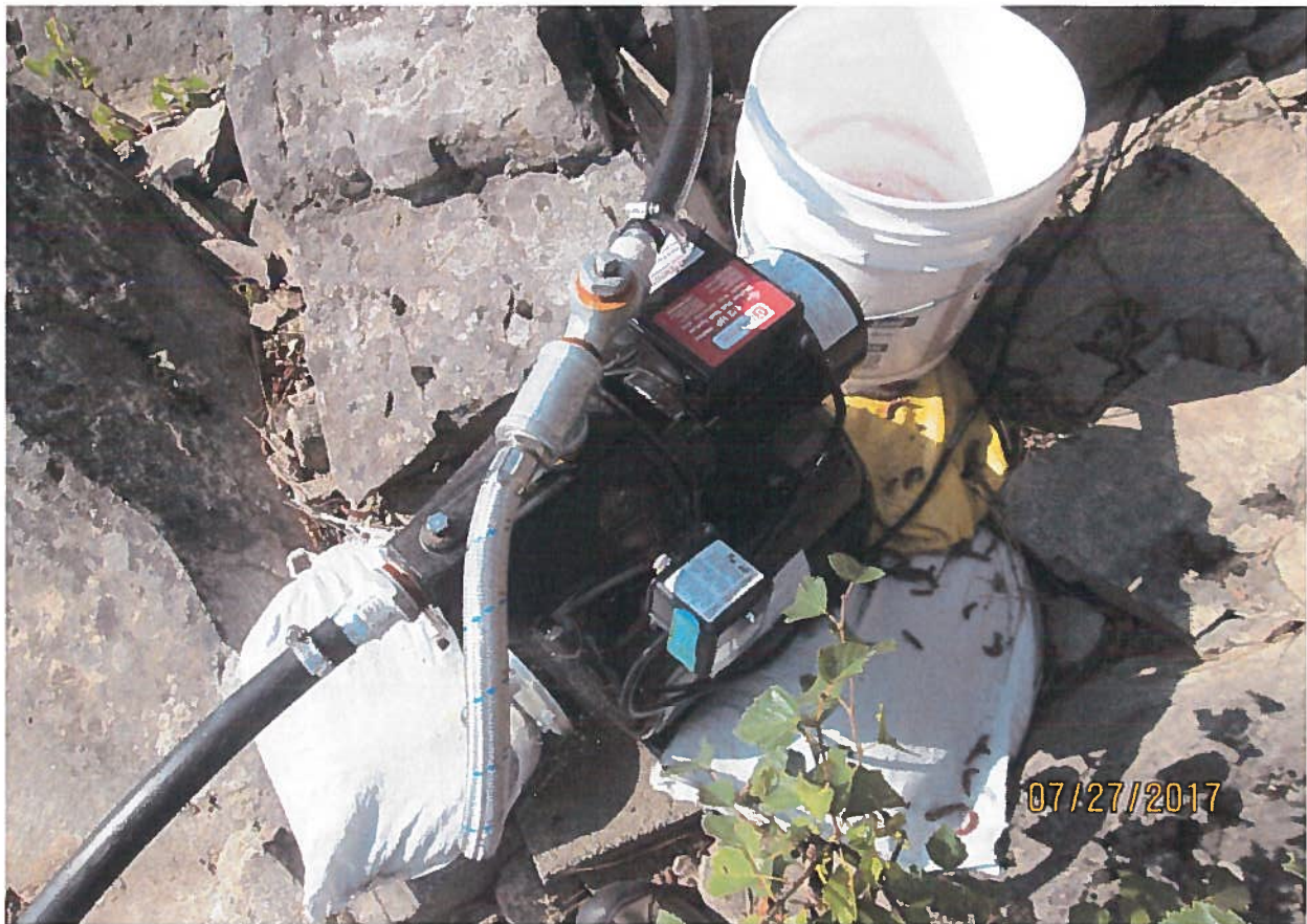
1/2hp Utilitech shallow well tank system pump.
