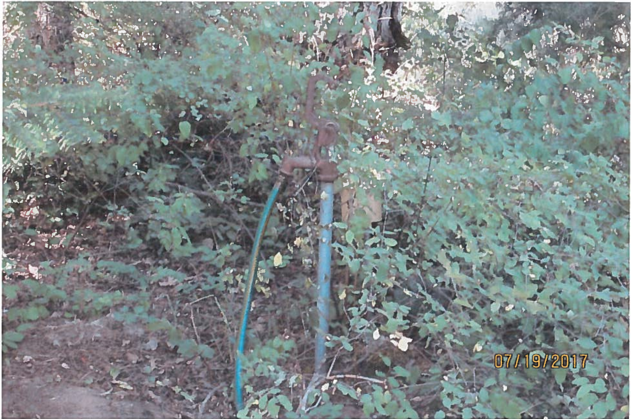
Frost free hydrant at bottom of hill where water was gravity fed to.
