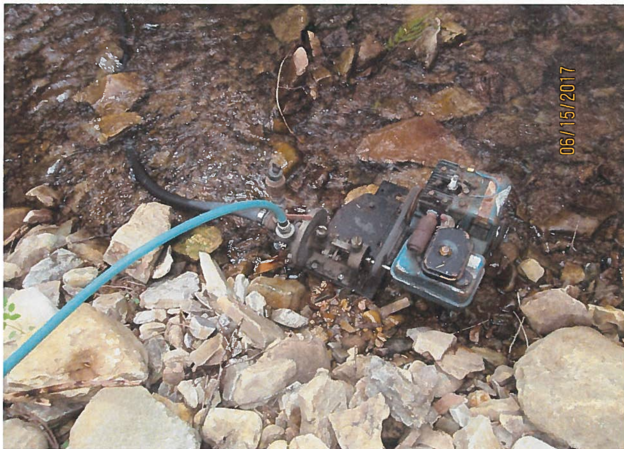
POD, unknown pump maker and pump size.
