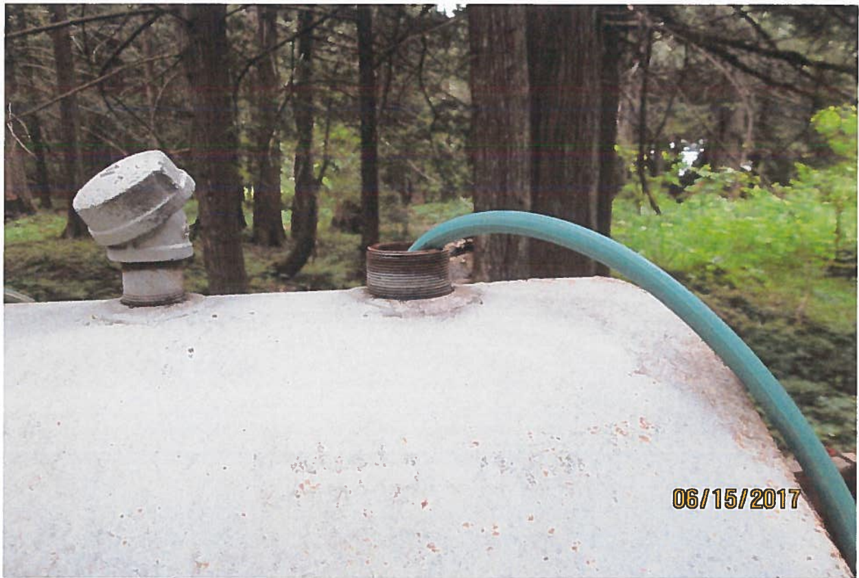
Applicant pumped from creek to 275 gallon storage tank. 5 gallon bucket test performed in 50 seconds.
