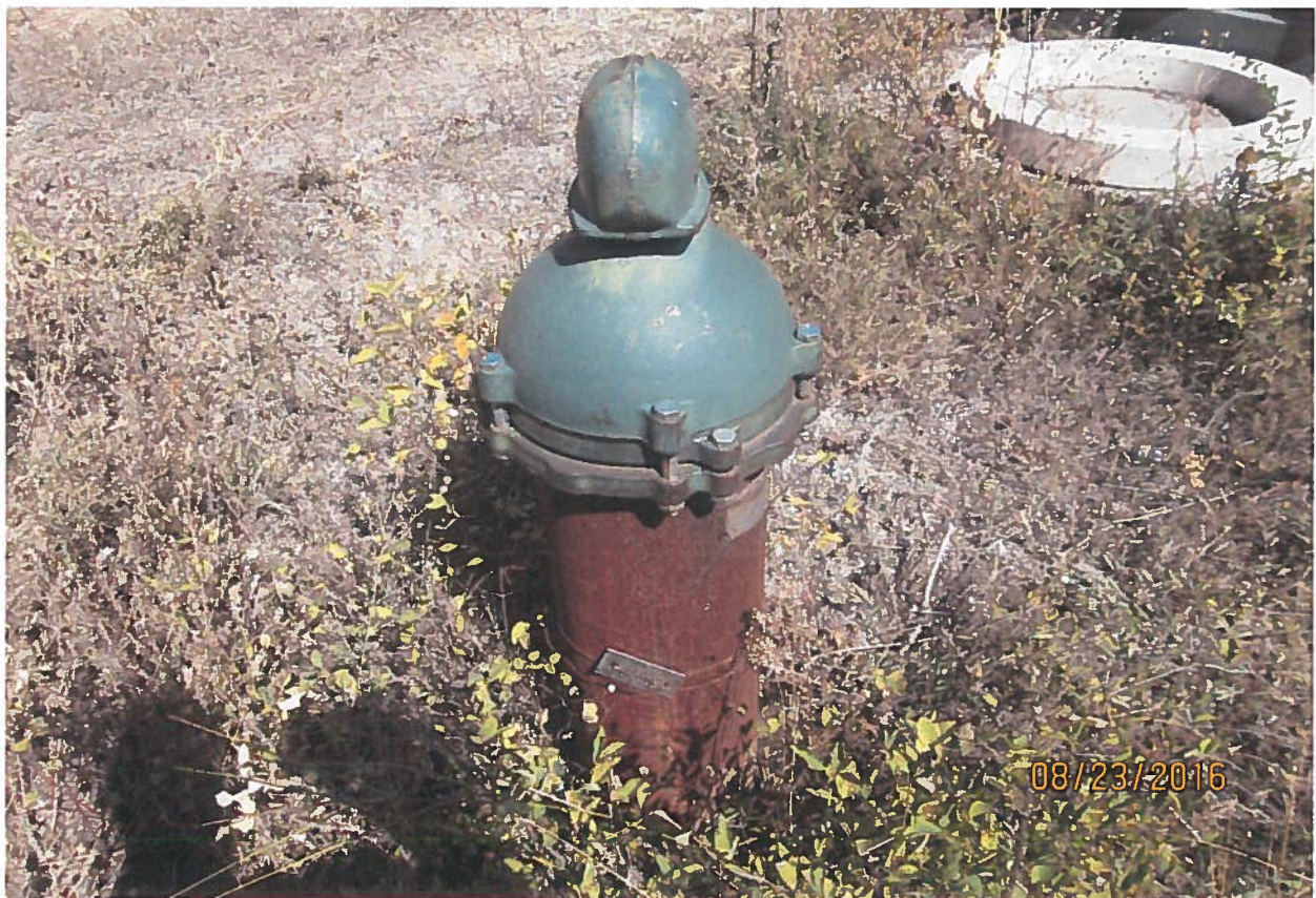
Well D0041376. 25hp Grundfos pump with diversion rate of 130 gpm.
