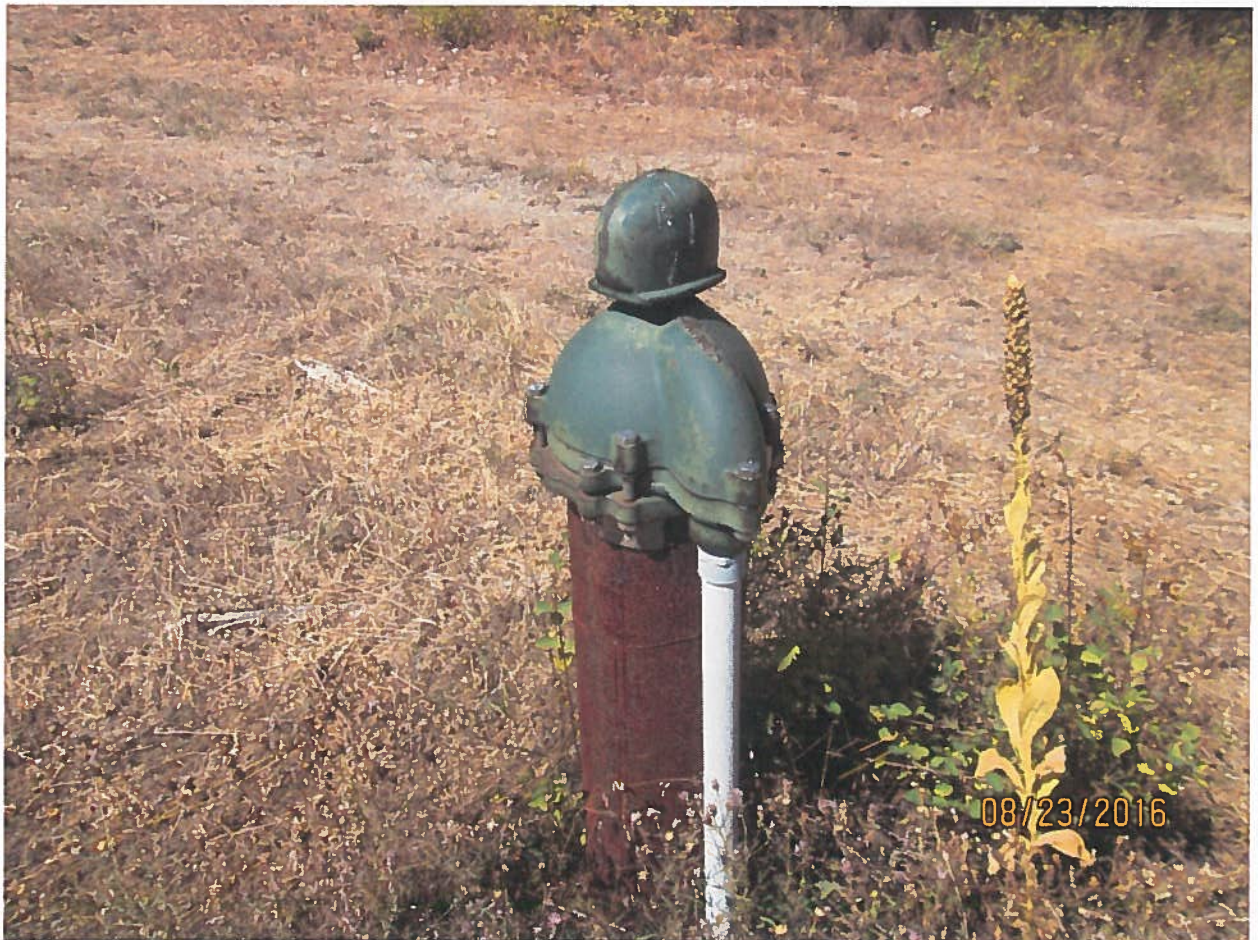
Well D0041375. 25hp Grundfos pump with diversion rate of 130 gpm.
