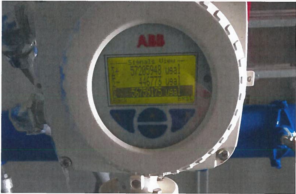
Plant Well #2 (West) Totalizer (12/29/2017)
