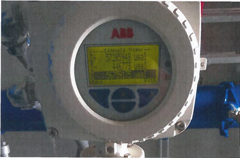
Plant Well #2 (West) Totalizer (12/29/2017)
