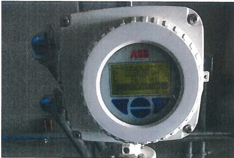
Plant Well #1 (East) Totalizer (12/29/2017)
