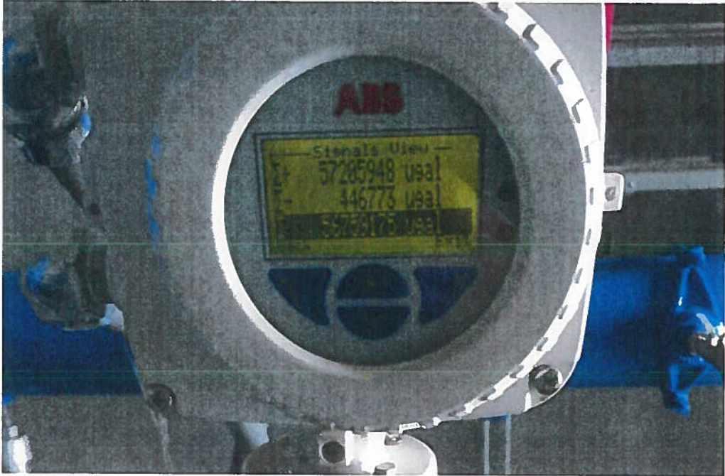
Plant Well #2 (West) Totalizer (12/29/2017)
