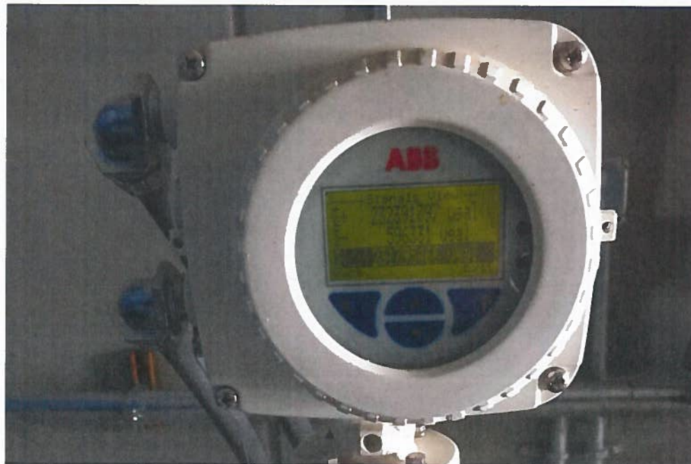
Plant Well #1 (East) Totalizer (12/29/2017)
