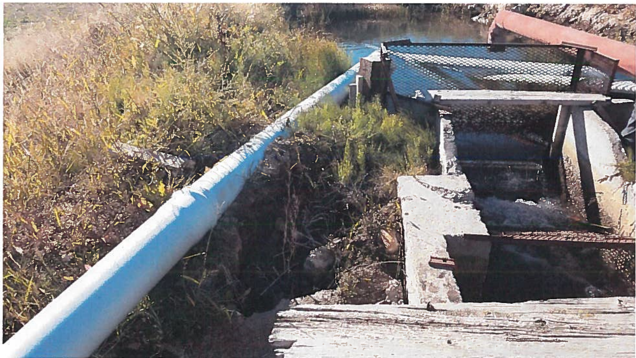
Picture 6. The Cipoletti weir between the collection pond and pumps that supply the buried pipe and ditches.
