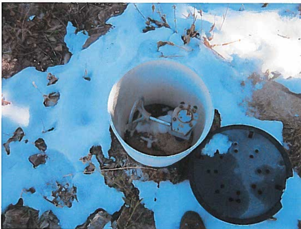
Figure 7: Valve used to divert water from pond to pump used for snowmaking.
