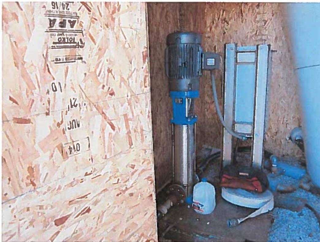
Figure 8: Vertical inline pump used for snowmaking.
