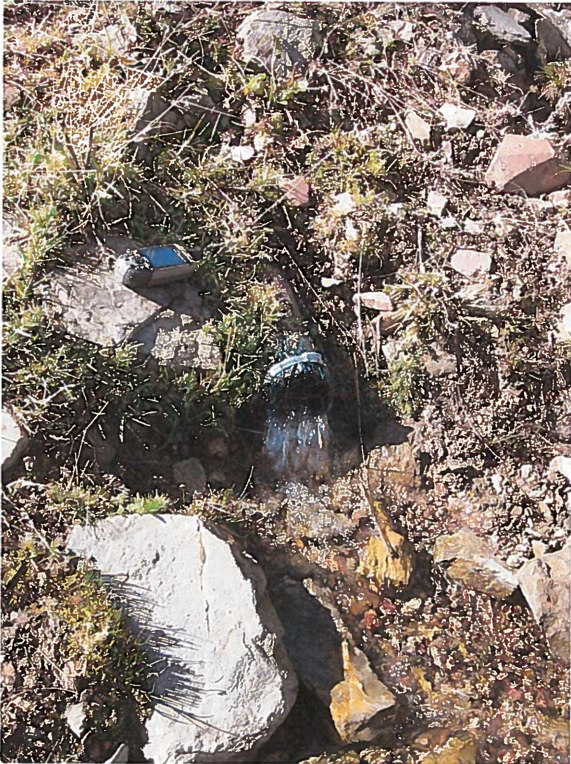
Figure 5: 1.5" pipe outlet into stream channel just west of the storage tank (note this is bypass flow). The actual conveyance system for 45-7745 is a 1.5" HDPE buried pipeline.
