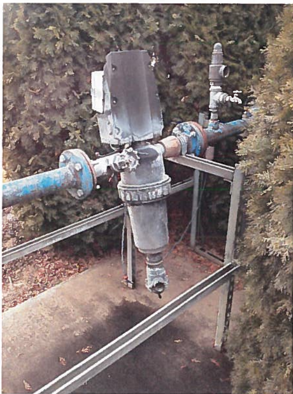
Figure 2 The 2" steel line from the well leading to the irrigation valves which are controlled by a RainBird timer
