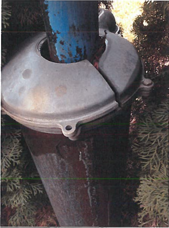
Figure 1 The 8" well providing water for irrigation of the landscaping surrounding the commercial buildings.
