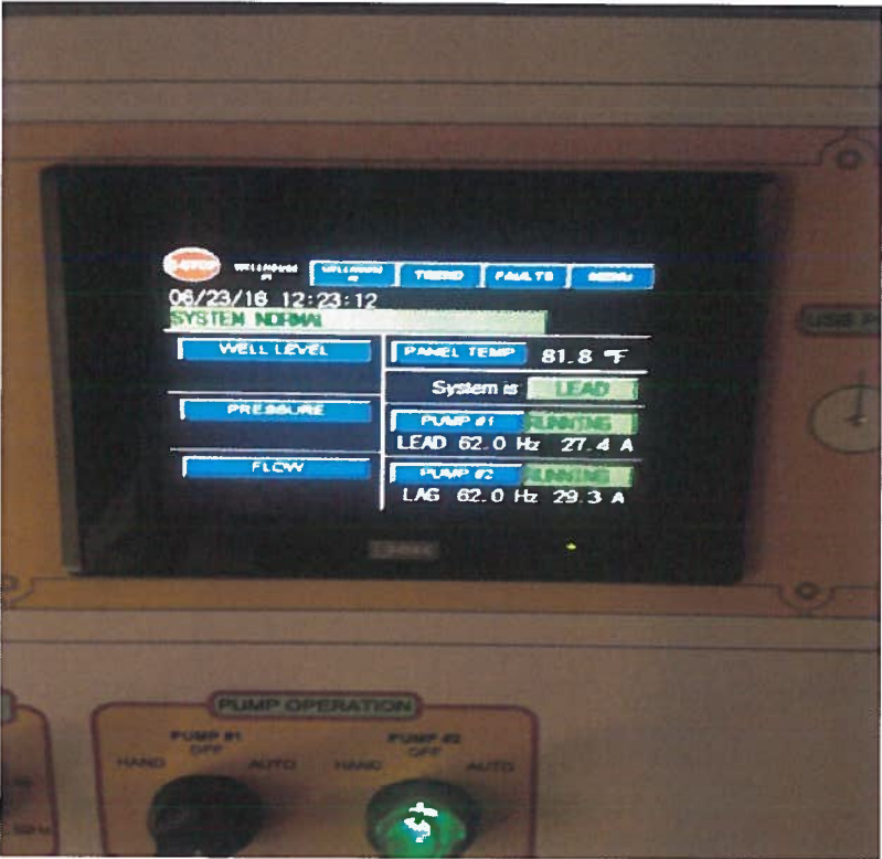
Well house # 2 both pumps maxed out Pressure dropped to 12 PSI
