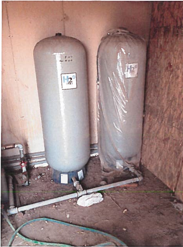
Figure 3 Storage tanks at the southern POD.
