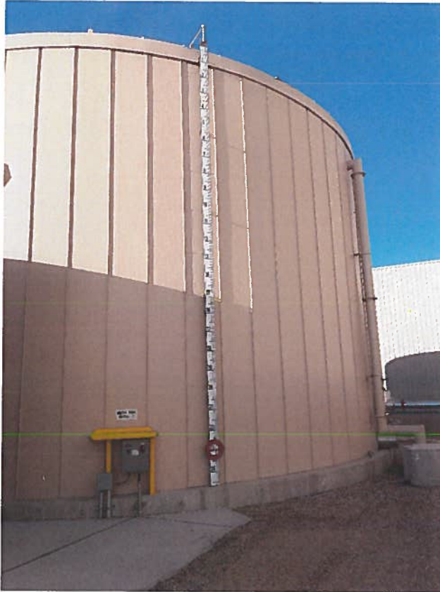
Figure 3 The 300,000-gallon storage tank where water is stored for fire protection use. The tank can be filled within a 24-hr period, so no storage component is required on the right. Water from the tank is distributed to the 5 hydrants on the property and to the internal sprinkler system inside the building.
