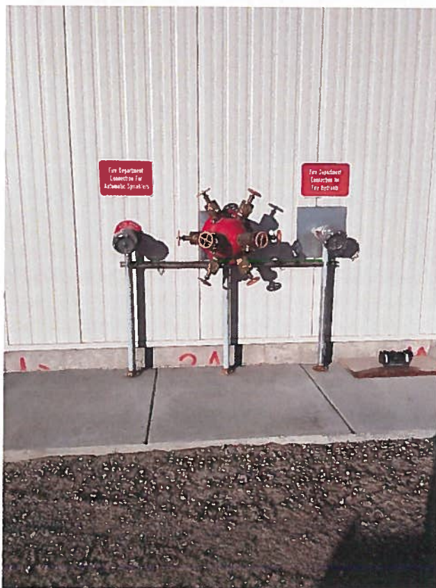
Figure 4 Connections at the pump house where the fire department can hook up to to fight fire.
