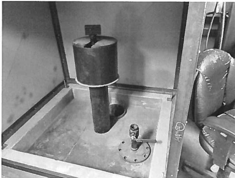
Figure 3 The well head located inside the warehouse in the NWSE QQ.
