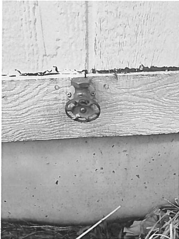
Figure 2 There are 5 hose bibs located throughout the property. Information submitted with the application suggests that maximum flow from these is around 3 gpm apiece.
