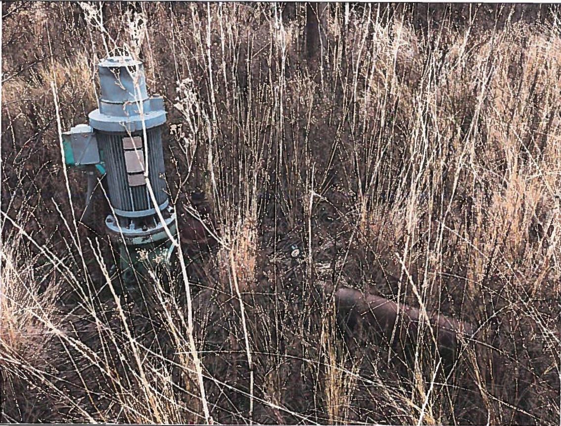
Well diverts water through a 10" mainline to risers for hand line sprinkler system.
