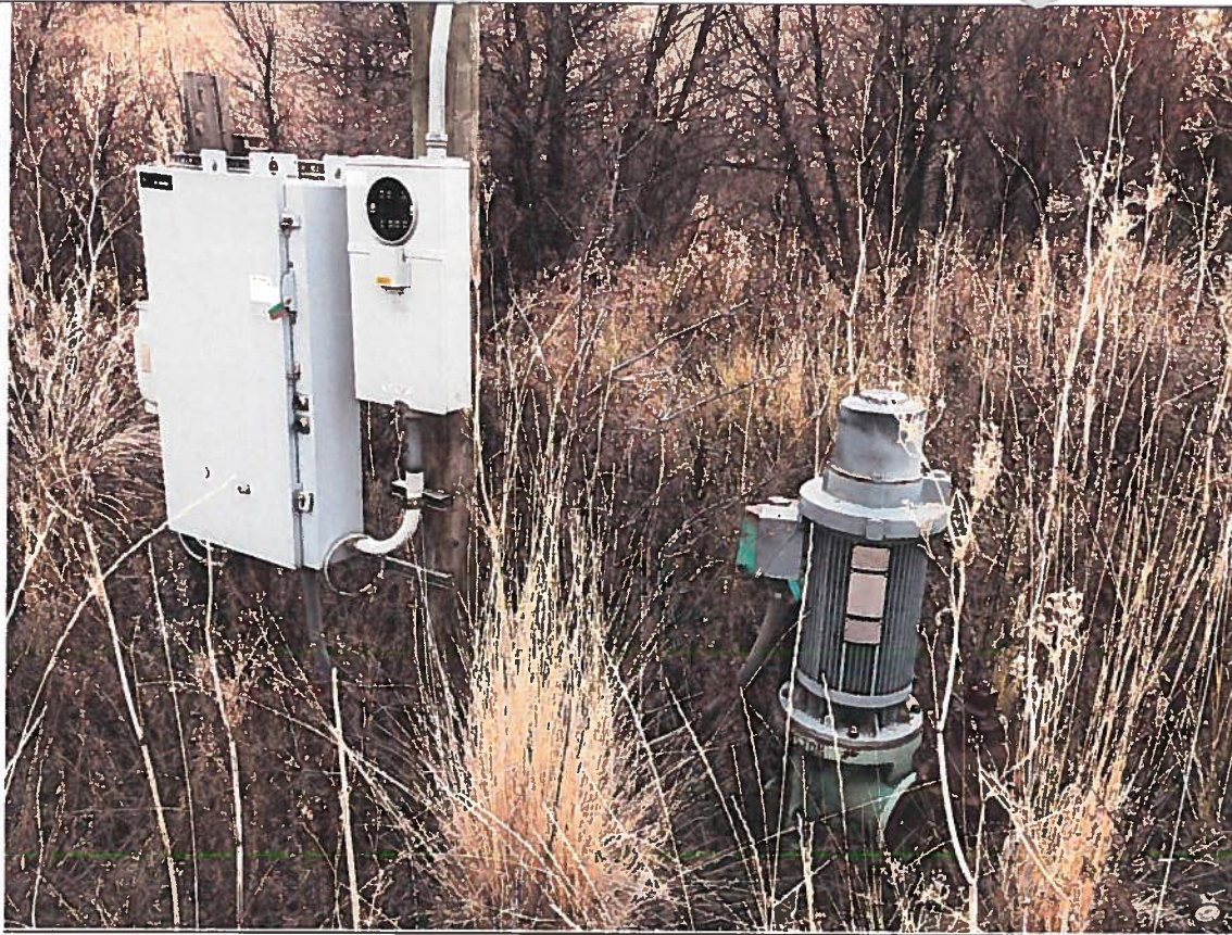
Well and power box
