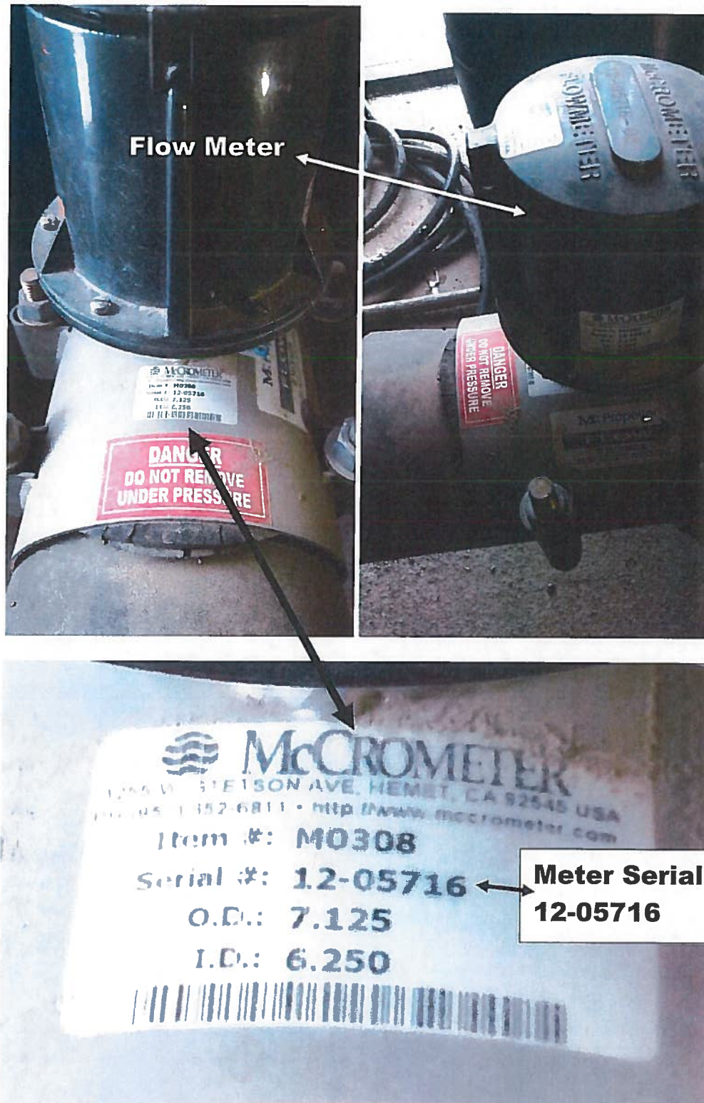
Flow Meter Tag for 40 Hp Submersible Hitachi Pump
