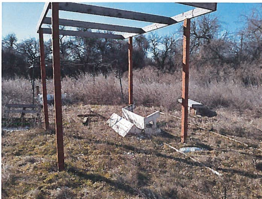
Figure 2 The seating and picnic area that has fallen apart since the project was abandoned.
