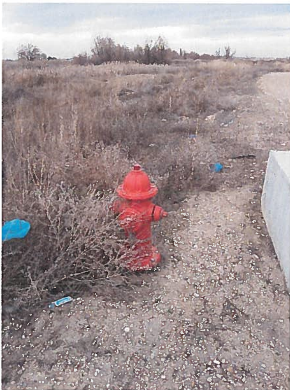
Figure 4 A hydrant located to the north of the pond. This is the only hydrant connected to this pond.
