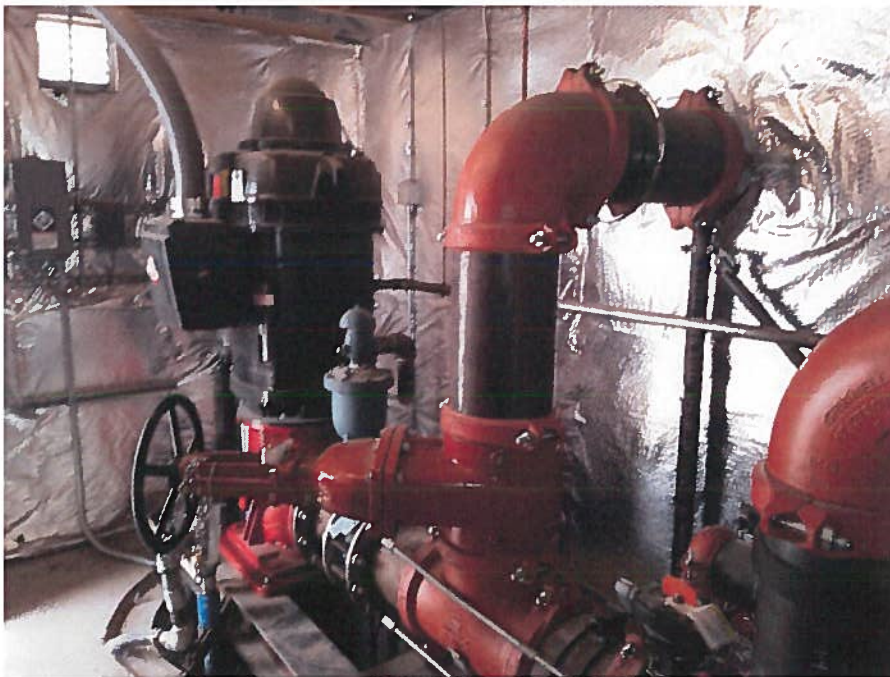
Figure 2 Inside the pumphouse just east of the pond. Water is pumped from the pond to a nearby hydrant and to charge the internal sprinkler system for the warehouse.
