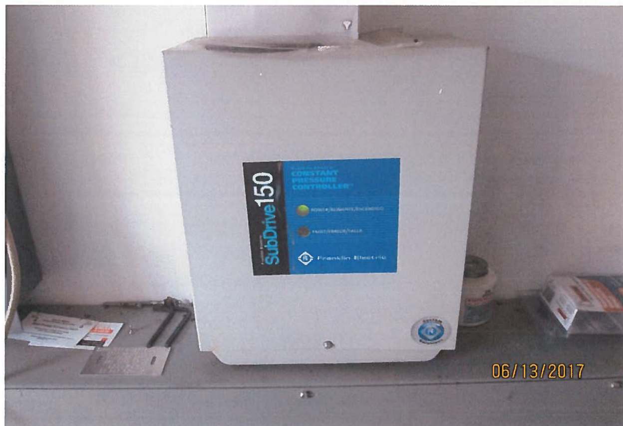
Franklin SubDrive 150, system was using a 3hp 3 phase pump.
