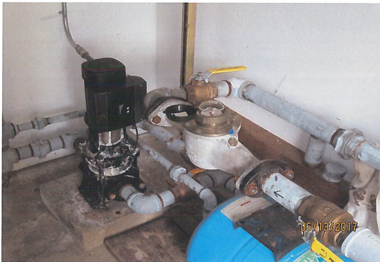
Flow meter on system with measurement of 24gpm.
