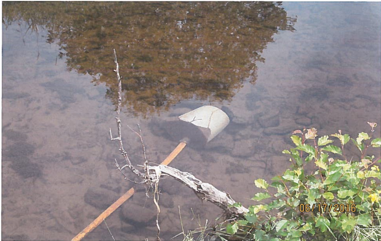
Screened intake at pump 2.
