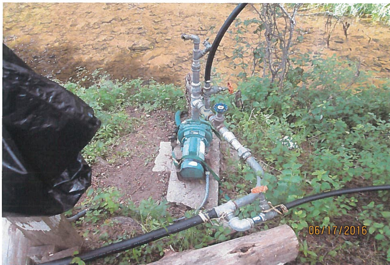
Pump 1. 2hp GE pump with diversion rate 20gpm.
