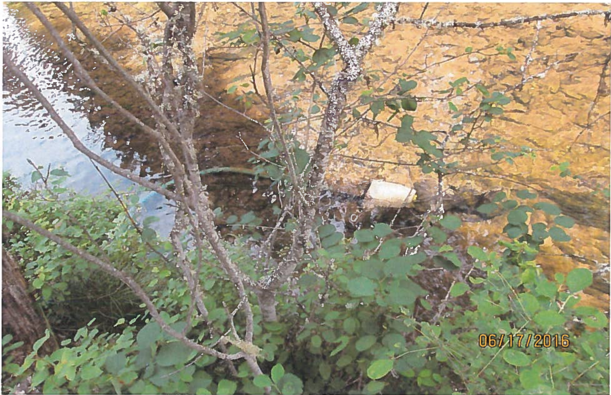
Screened intake at pump 1.
