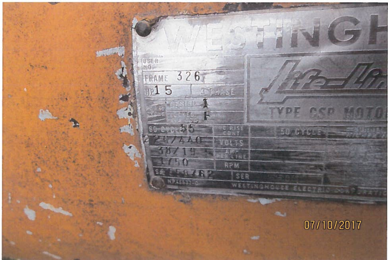
15hp Westinghouse pump.
