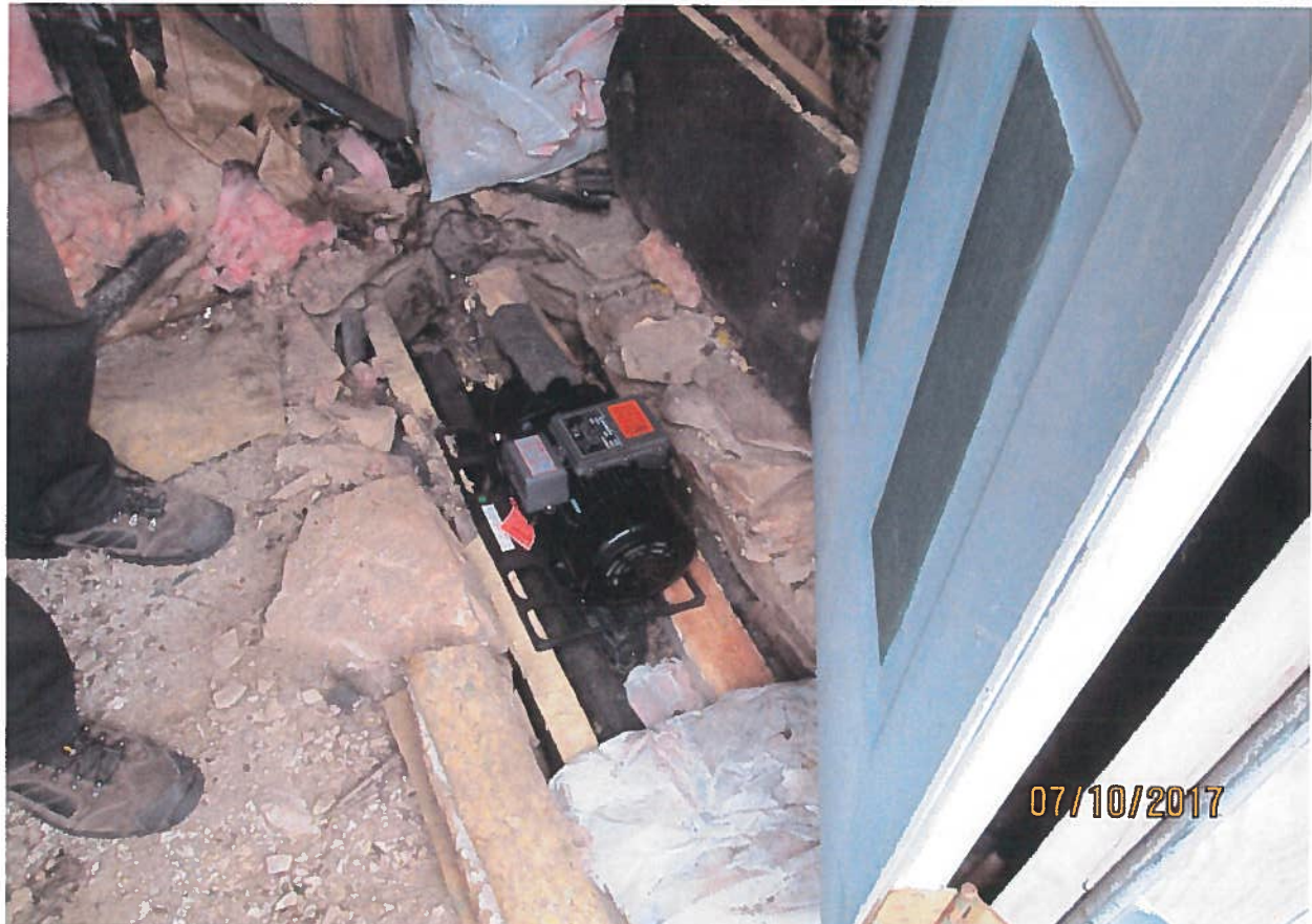
3/4hp pump in pump house. Measured flow from pump was 19gpm.
