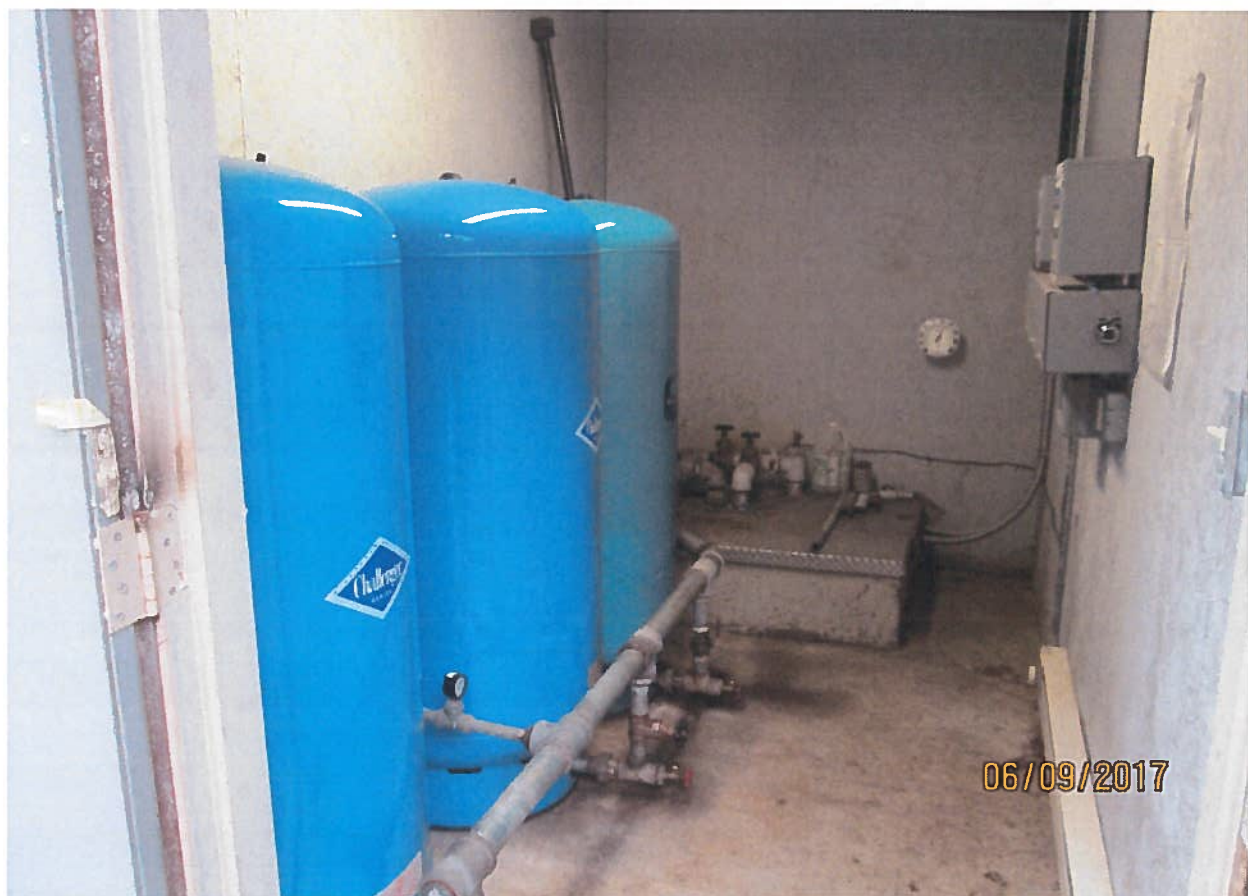
Inside of pump house. 3,000 gallon vault under floor.
