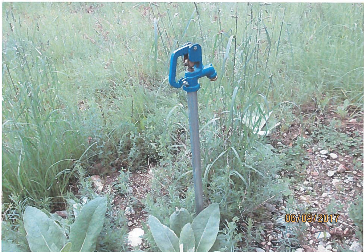
Frost free hydrant stub-in.
