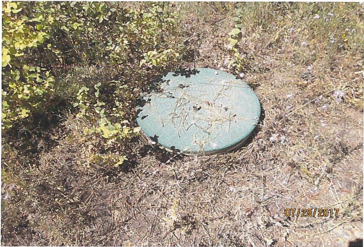
3,000 gallon cistern. Unable to perform any measurement because water was pumped directly into storage tank.
