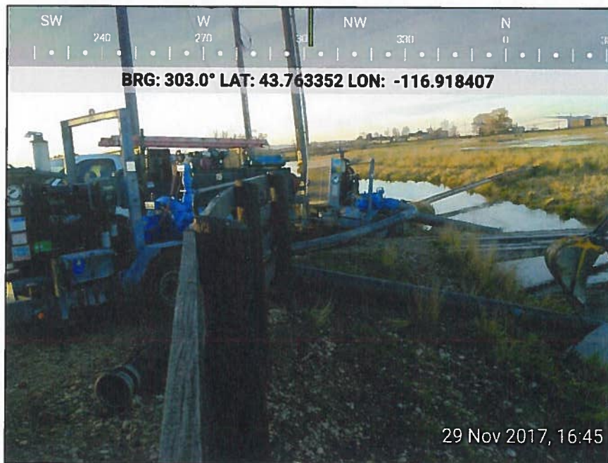
Figure 4: Pump 2 in position in foreground with Pump 1 in background.
