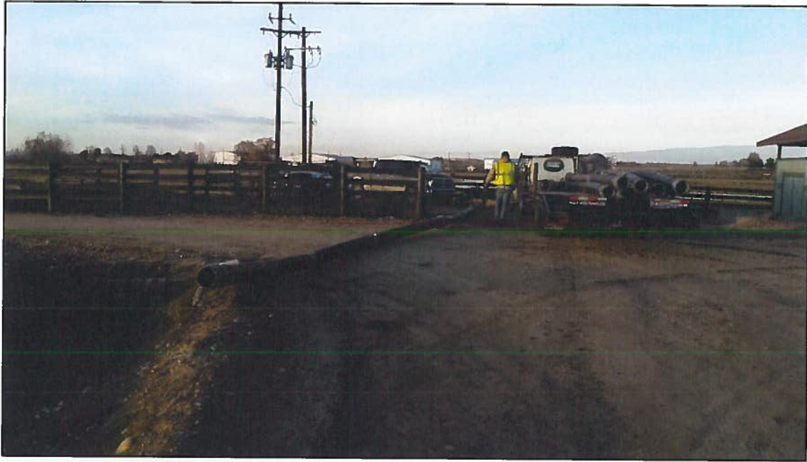
Figure 5: Pump 2 discharge pipe set to discharge into ditch feeding Rest Pond area.
