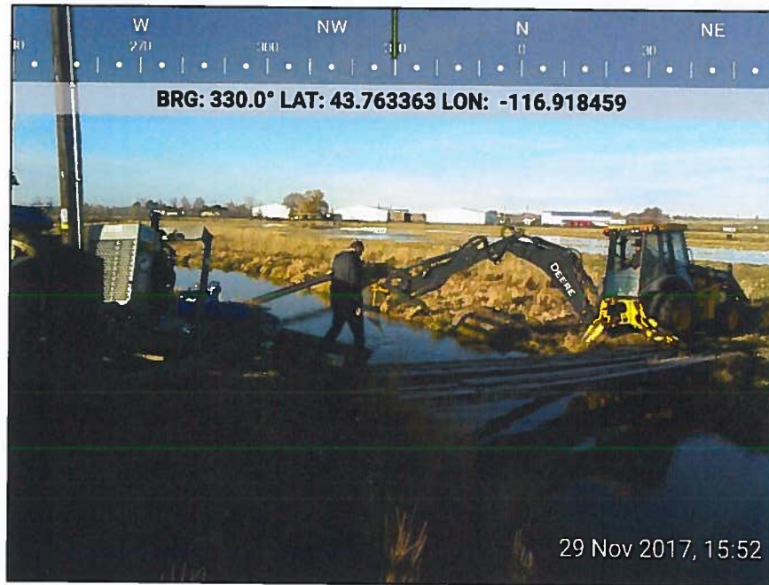
Figure 1: Pump 1 diverting from Sand Hollow Creek.
